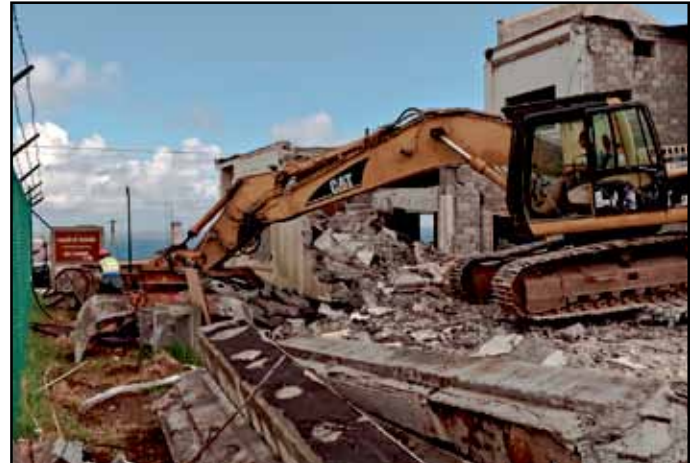
Building T-252, Lajes' first American Forces Network building, was torn down in November due to its old age and inconvenient off-base location upon Santa Rita Hill.. (Photo by Lucas Silva)
