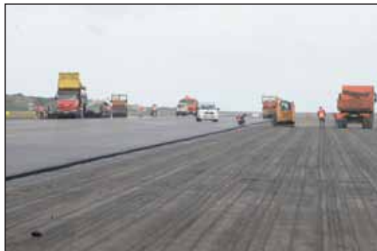
The Lajes flightline is currently undergoing pavement repair, and the 65th Civil Engineer Squadron is in charge of the project. (Photo by Guido Melo)
