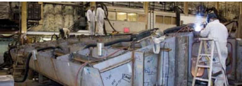
Workers at the General Dynamics-Bath Iron Works shipyard in Bath, Maine, weld together pieces of an inner-bottom unit for the future USS Zumwalt (DDG 1000). (Photo courtesy General Dynamics)
