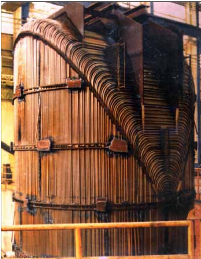
Figure 9.4 Recirculating steam generator tube bundle
