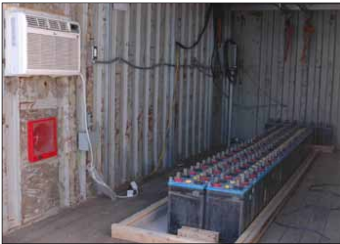
Figure 7.14 Battery bank for dc fire tests
