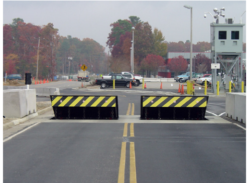
Changes to the DBT have warranted an increase in physical security, including enhancements to vehicle barriers.
