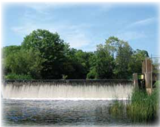
The Winnicut River Dam in the spring of 2009, before the project began. Credit: NOAA
