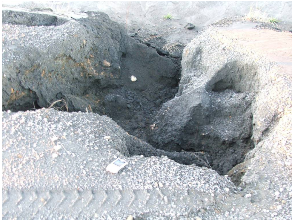
Figure 16. Erosion Along Crest of Dredge Cell, 2009
