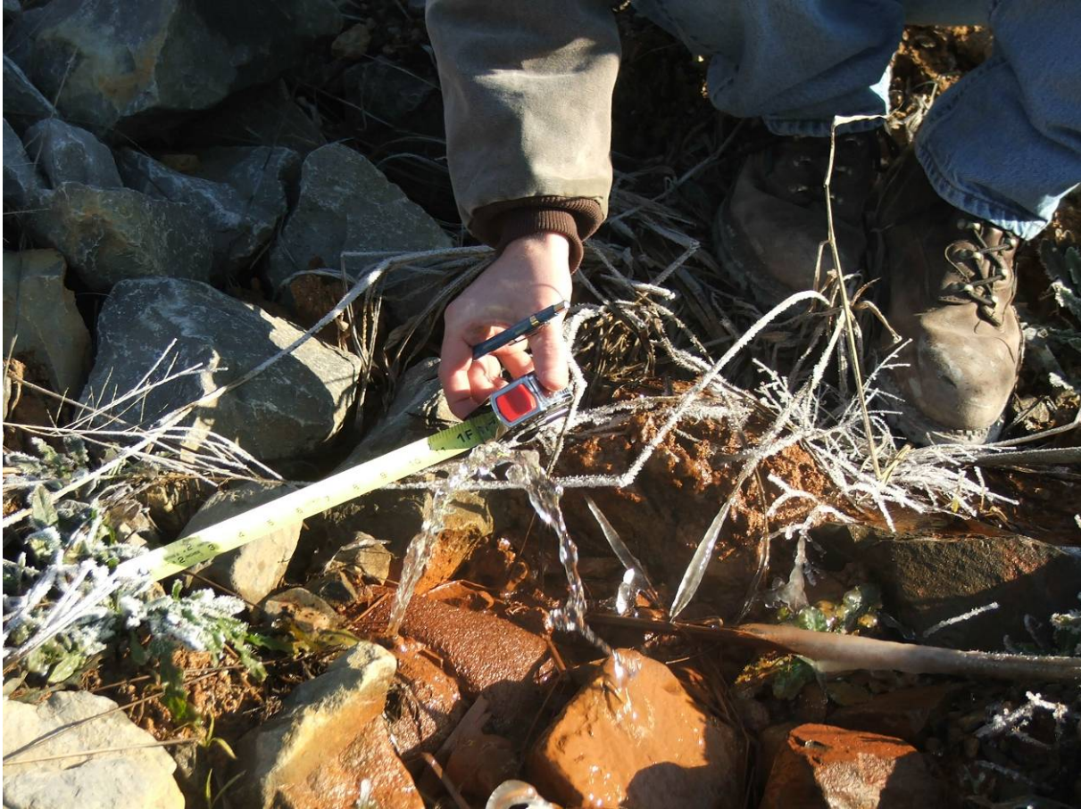
Figure 21. Seepage/Excessive Pore Pressures along Scrubber Road, 2009
