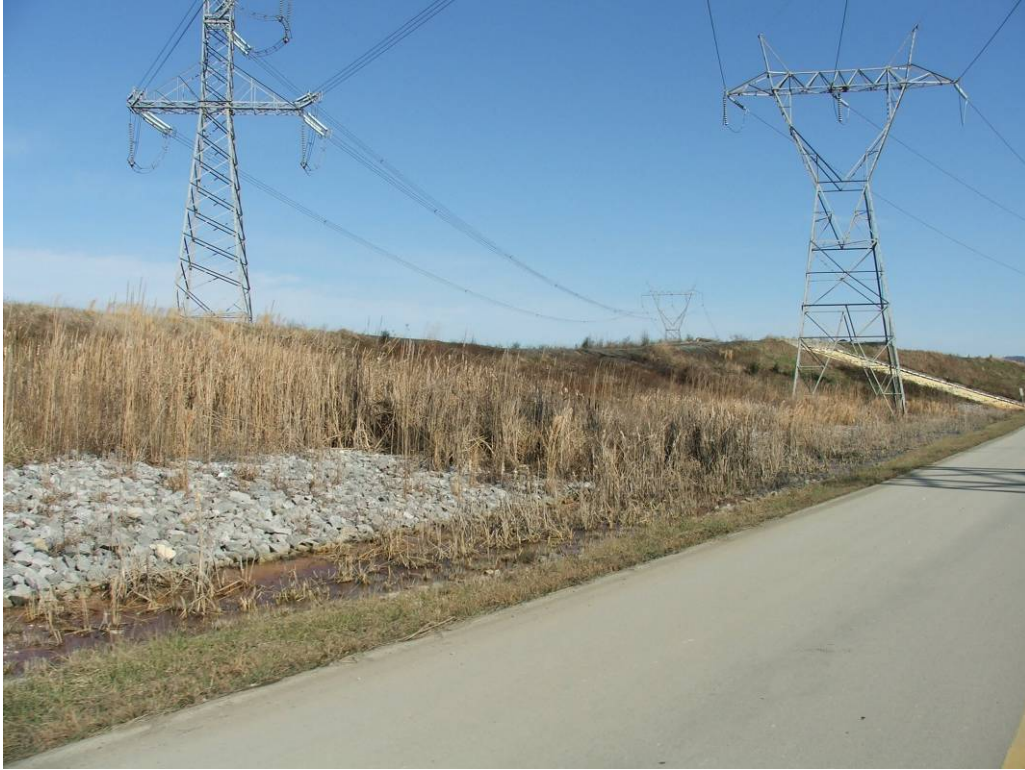
Figure 19. Ditch/Seepage Conditions Scrubber Road, 2009
