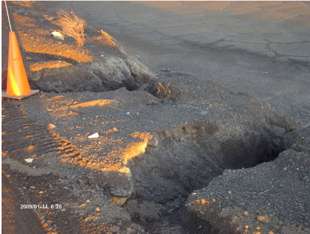
Figure 15. Erosion Along Crest of Dredge Cell, 2009
