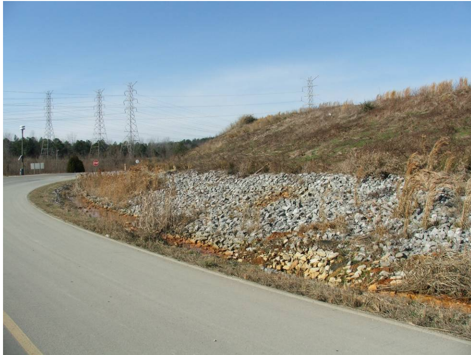
Figure 17. Ditch/Seepage Conditions along Scrubber Road, 2009
