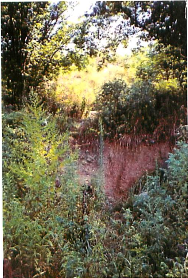
View showing sloughing on dike.
