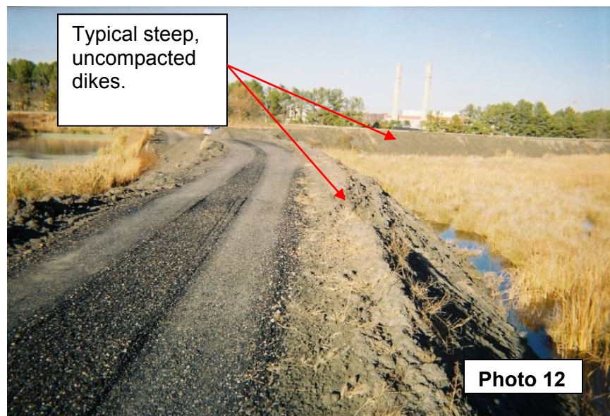
Photo 12. Bottom Ash Pond. Typical Steep Uncompacted Dikes.
