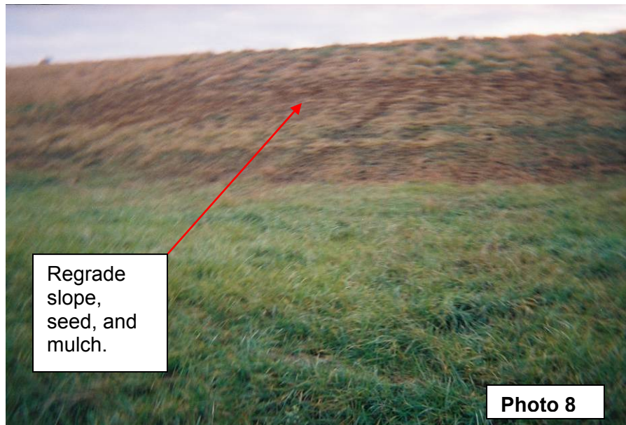
Photo 8. Slough area beside Northeast Seepage Collection.
