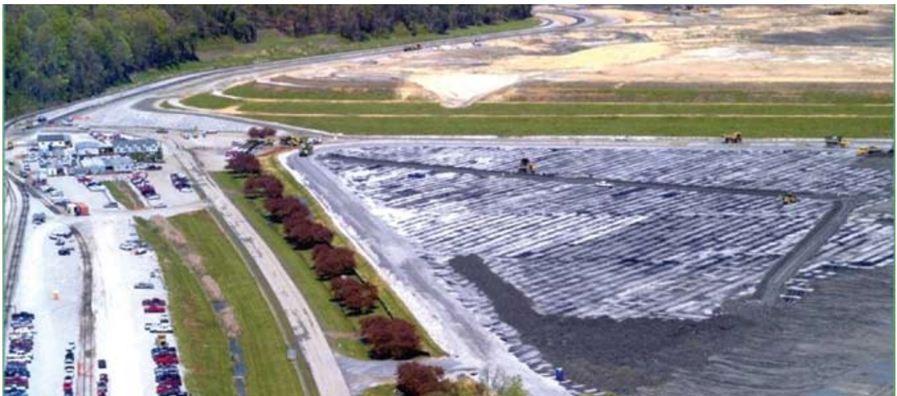
Ash removed from the channel is brought to this temporary storage area to dry.
