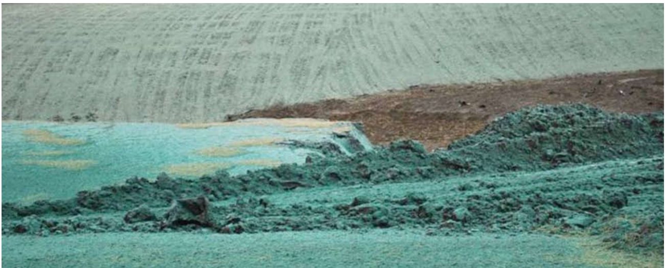
TVA has applied Flexterra to more than 290 acres since January to reduce airborne dust from the site.
