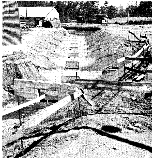
FIGURE 126.—Concrete supports for ash sluice piping in open trench. Note 12-inch corrugated pipe sleeves (background) through which ash pipes were carried under yard tracks.
