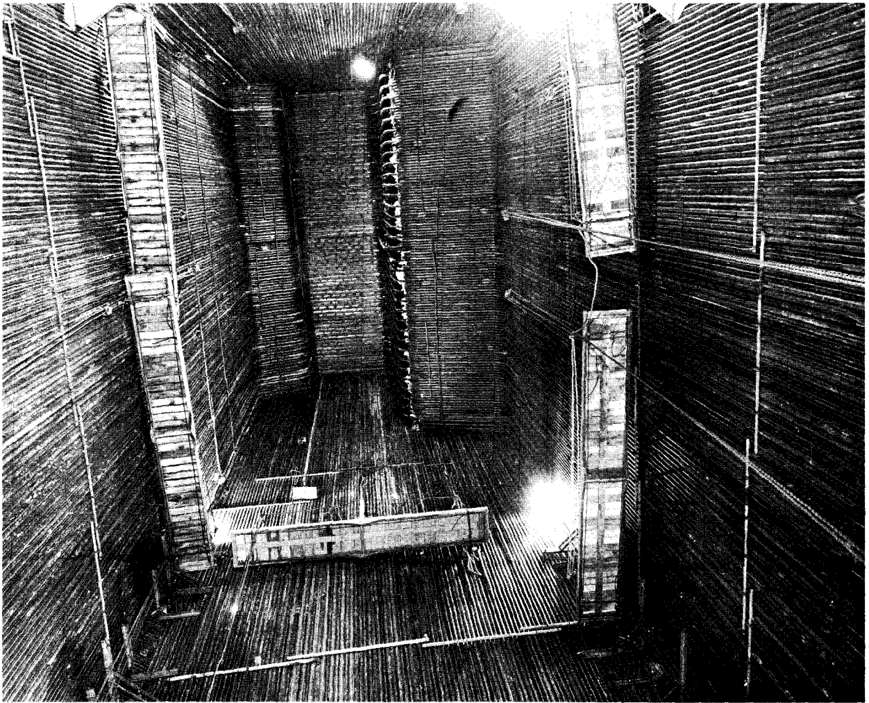
FIGURE 116.— Inside unit 1 boiler looking up from ash hopper showing tubing for furnace water walls, superheater and reheater elements.
