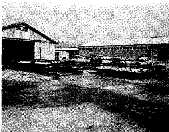
FIGURE 153.—Gas duct panels, made up of pieces from the old duct, cut, punched, and tack welded, were placed on outdoor tables to be assembled with some new panel pieces, beams, and stiffeners.
