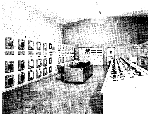
FIGURE 58.—Electrical control room in control building. From left to right—recording instrument board, operator's desk, motor-generator set board, benchboard, and main instrument board.
