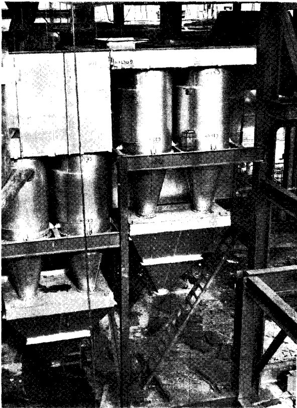
FIGURE 125.—Unit 1 fly ash collectors. There are 16 cyclonic elements assembled in a steel housing with two assemblies per unit.
