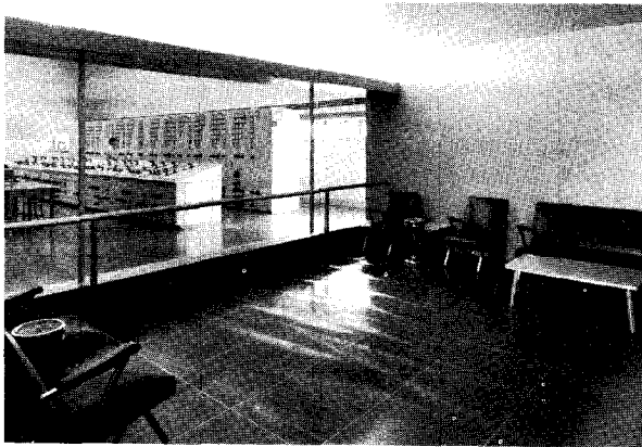
FIGURE 57.—Visitors lobby in the control building. This room was provided to afford visitors a view of the electrical control operations.
