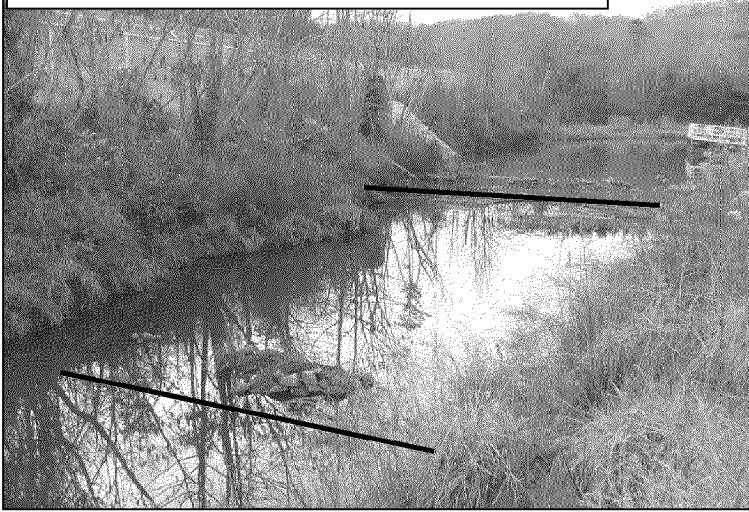
Fig. 11 Breached Check Dams
