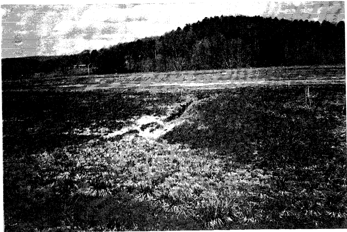
Figure 2. Area of erosion in perimeter ditch in northern corner of Dredge Cell 2.
