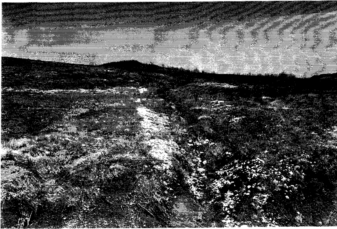
PICTURE 1- GULLIES AND ERODED AREAS ALONG NORTH DIKE
