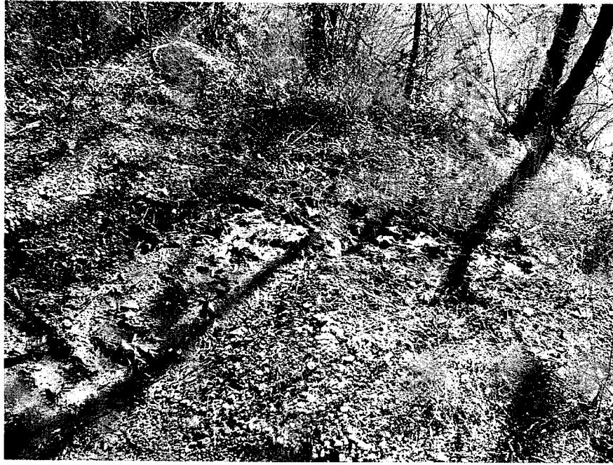
Photo 9. Dike slope erosion.
