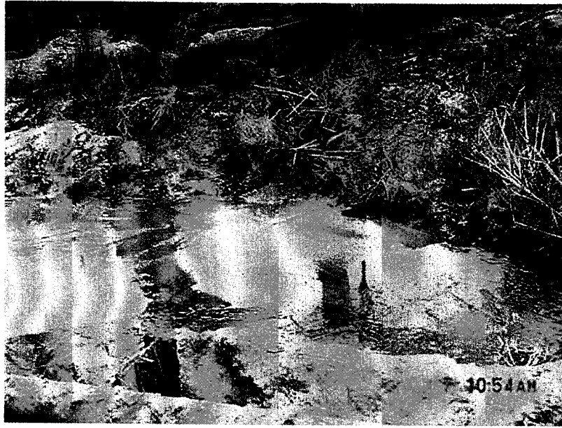
Photo 1. Leak in the toe of the slope of dredge cells 2/3
