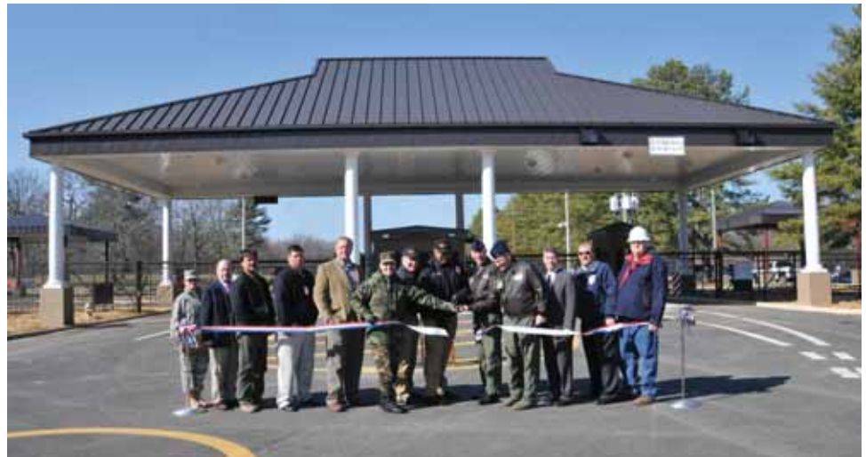
Above, renovations at the Fitness Center included repaving the outside entry ways, adding new canopies, a new HVAC system, a renovated lobby, a new weight room and landscaping. Right, Arnold AFB's Main Gate construction project included reconfiguration of the entrance from Wattendorf Highway, a new entry facility and entry booth.
