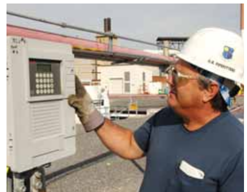
R. A. Millen, an ATA pipefitter, checks fuel flow at the AEDC fuel farm.
