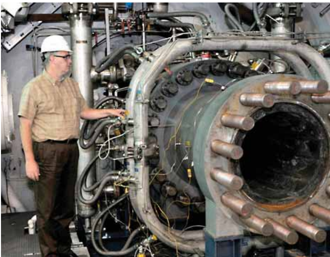
Dr. Lynn Seburn, an ATA facility systems analysis team engineer, inspects the cooling water lines of the combustion air heater at the Aerodynamic and Propulsion Test Unit (APTU) prior to a test run.
