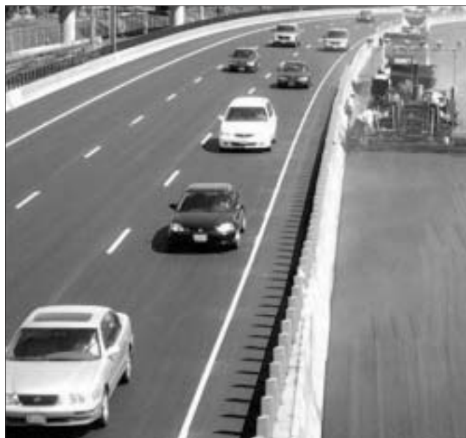
Figure 2 – Crews work without interruption on I-84 (Banfield Freeway), physically separated from traffic
