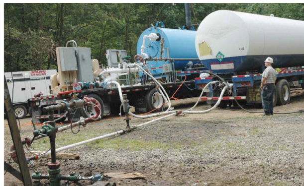
Crew member monitoring CO 2 injection operations during the injection phase of the "huff n' puff" test at the Sickafosse-Morris well
