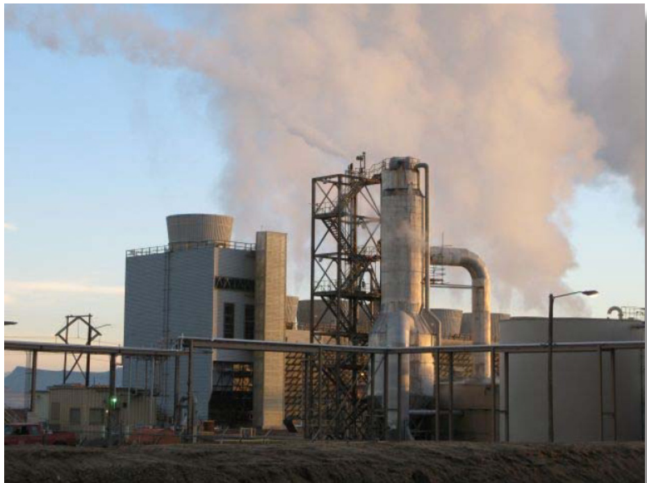
Air2Air Validation Cell in Operation Next to Wet Only Cooling Cells
