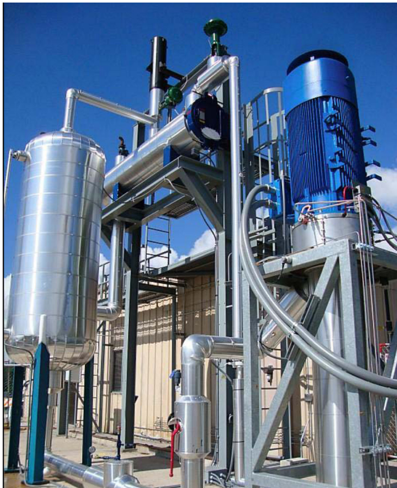
Liquid CO 2 pump test loop
