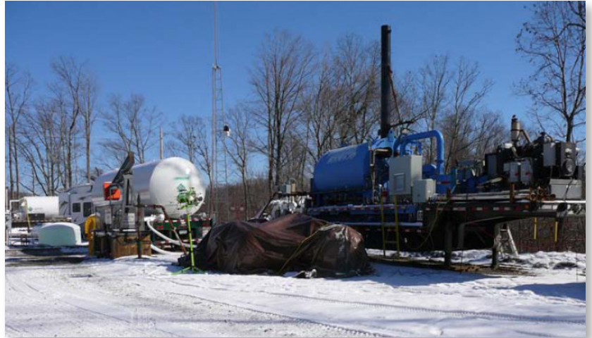
Injection operations at the Central Appalachian Coal Seam site in Russell County, Virginia.
