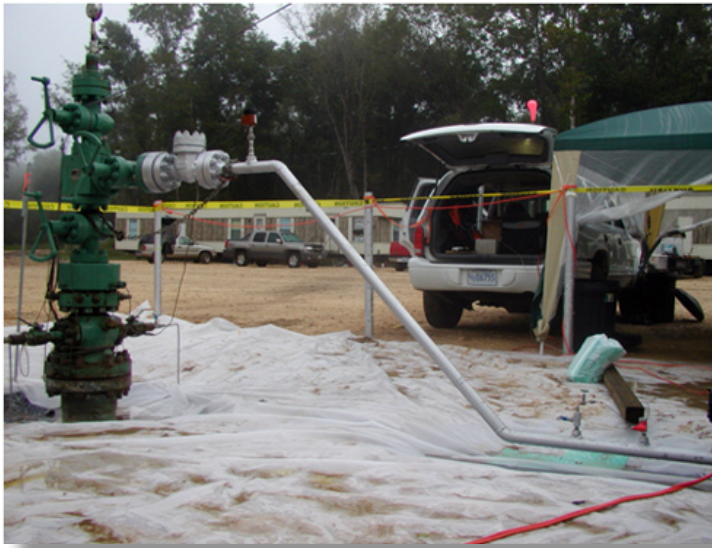
Figure 1: Perfluorocarbon tracers in a syringe pump located in the back of the NETL van are being added to carbon dioxide as it is injected underground at the Frio saline reservoir sequestration test site near Houston, Texas.
