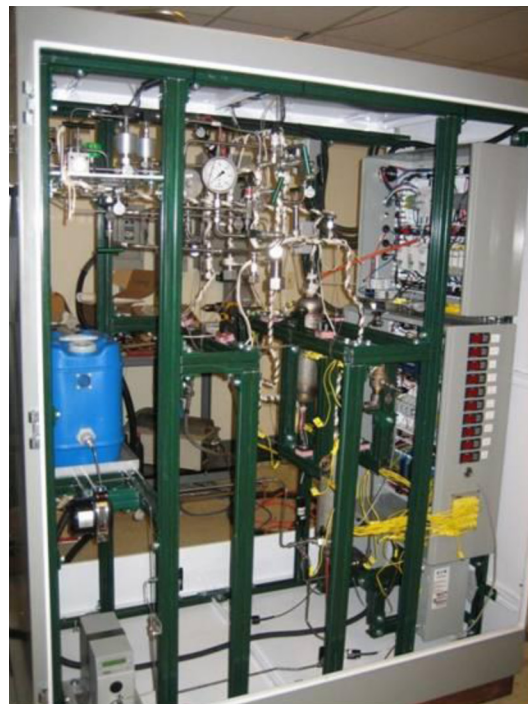
Figure 2. TDA's Gas conditioning skid.
