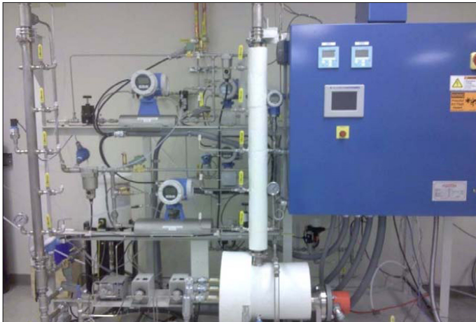
Akerman's Closed-Loop Reactor for Carbon Capture Testing.
