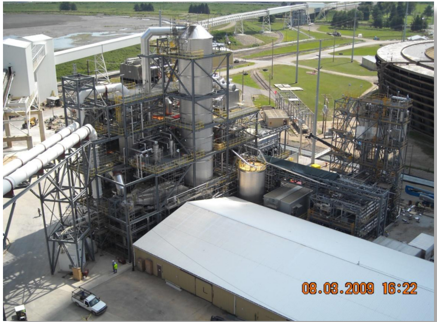
Figure 1. Chilled Ammonia CO 2 Capture Process Validation Facility
