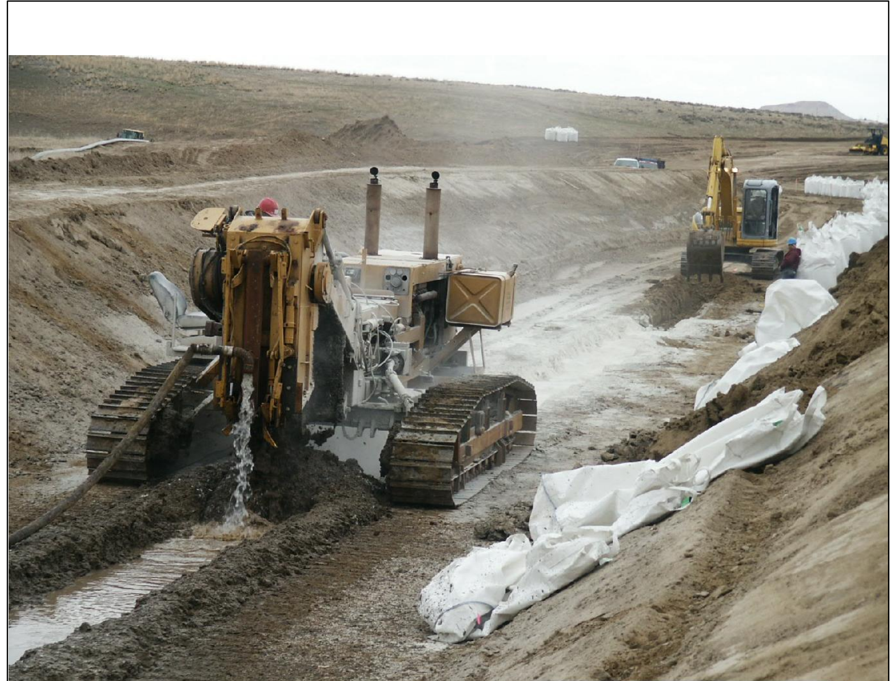
BELLE AYR MINE CBW INSTALLATION (2004)
