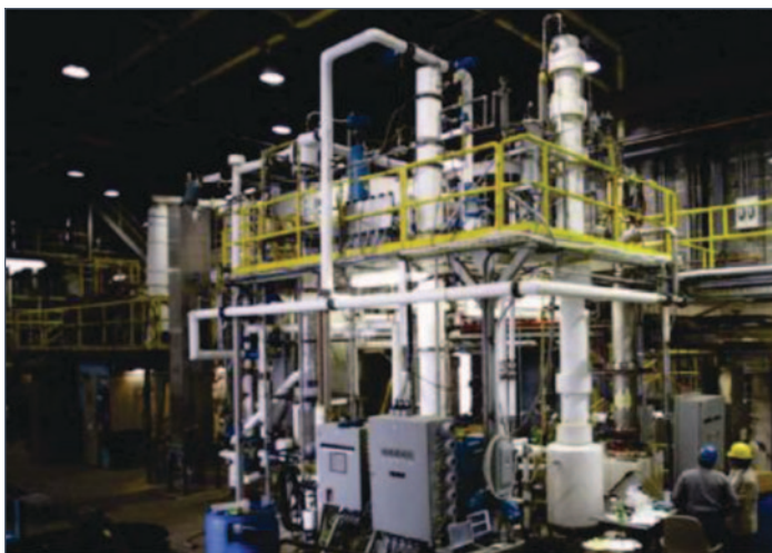
Figure 1: UNDEERC Post-Combustion CO 2 Capture Test Facility
