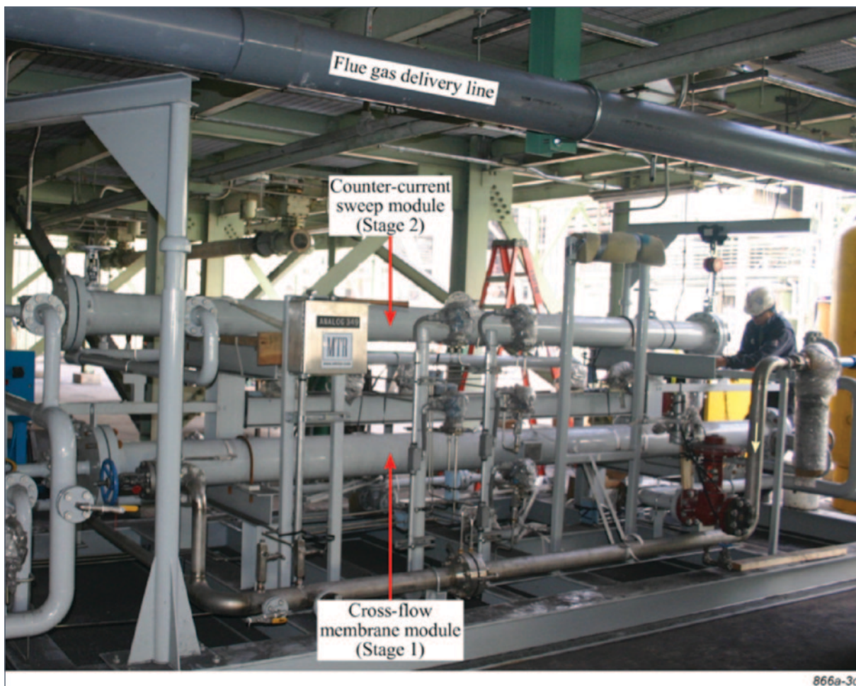
Figure 4: Membrane Skid Used for Pilot-Scale Slipstream Testing at the APS Cholla Power Plant
