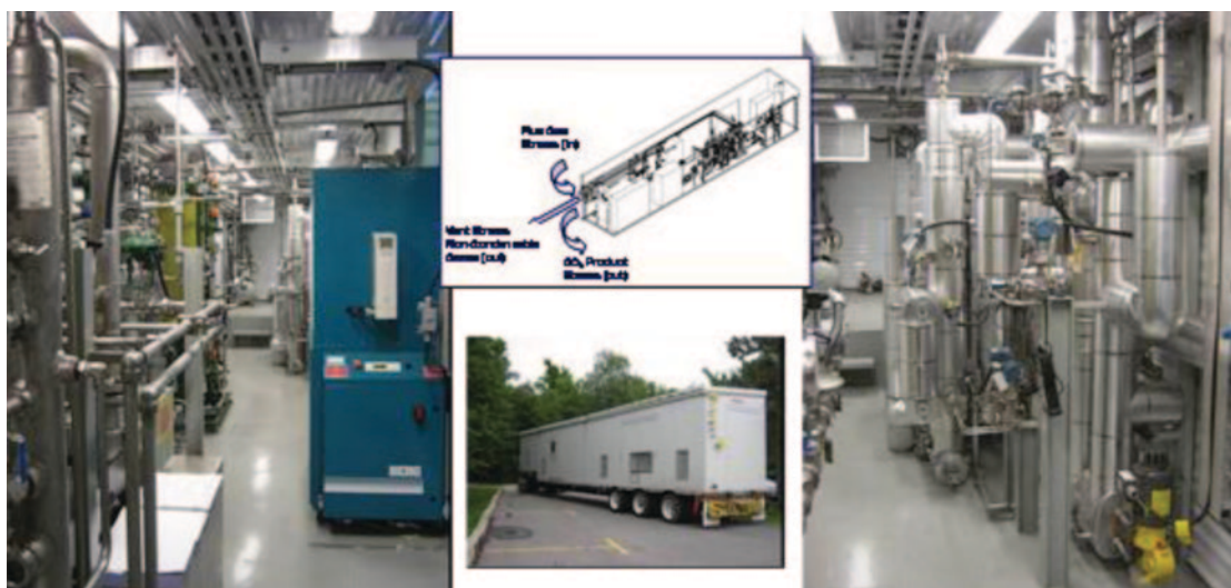
Figure 2: CanmetENERGY's CO 2 Capture and Compression Unit
