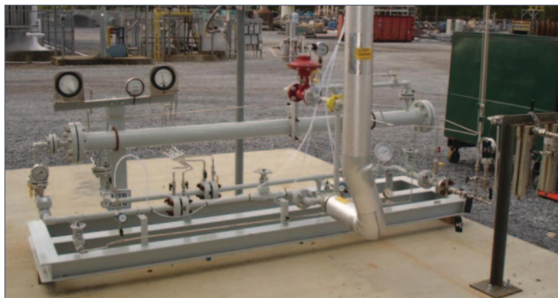
Figure 3: MTR Membrane Test Skid at the National Carbon Capture Center
