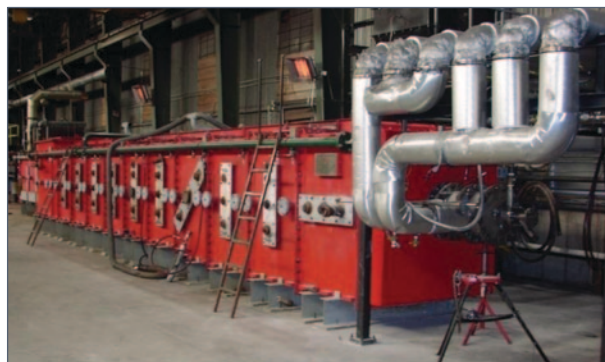
Figure 2: Pilot-Scale Combustion Facility (L1500)
