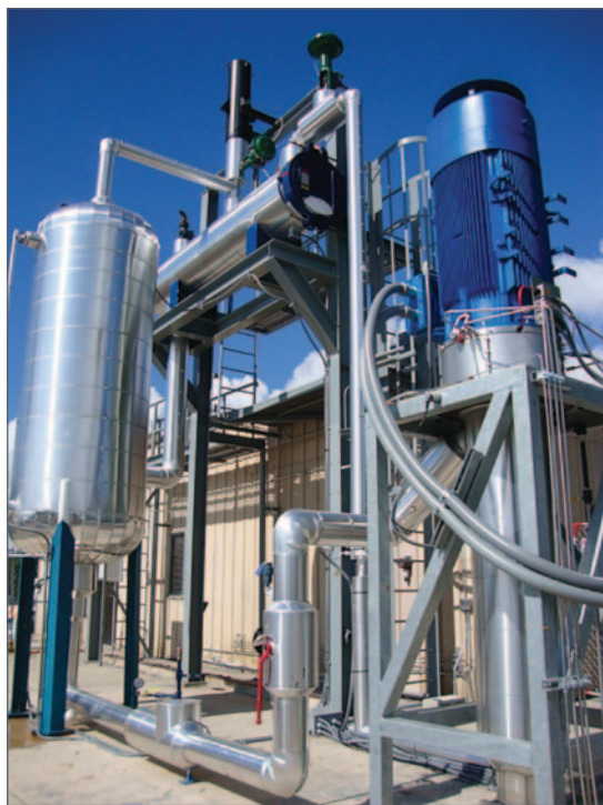
Figure 4: Existing Liquid CO 2 Pump Loop Constructed at SwRI
