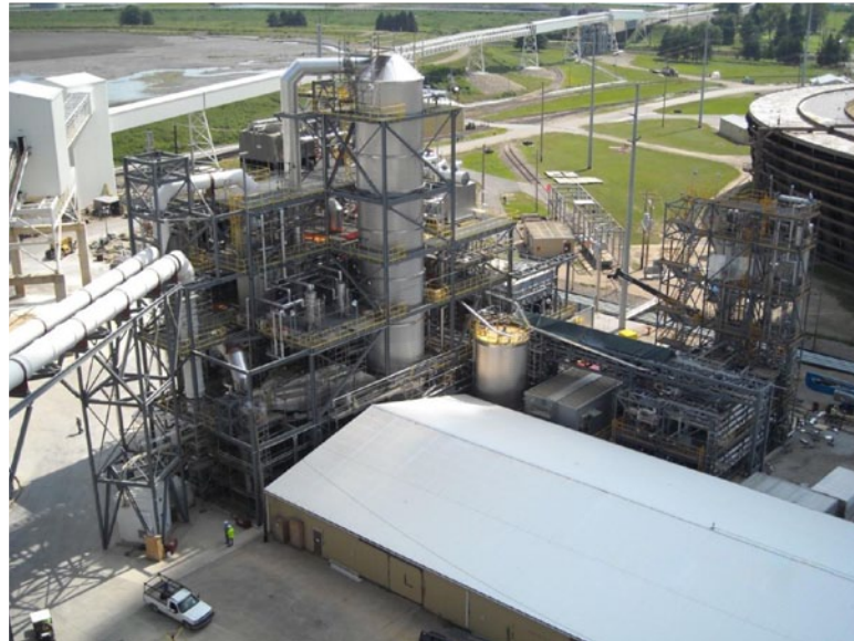
Figure 1. Chilled Ammonia CO 2 Capture Process Validation Facility
