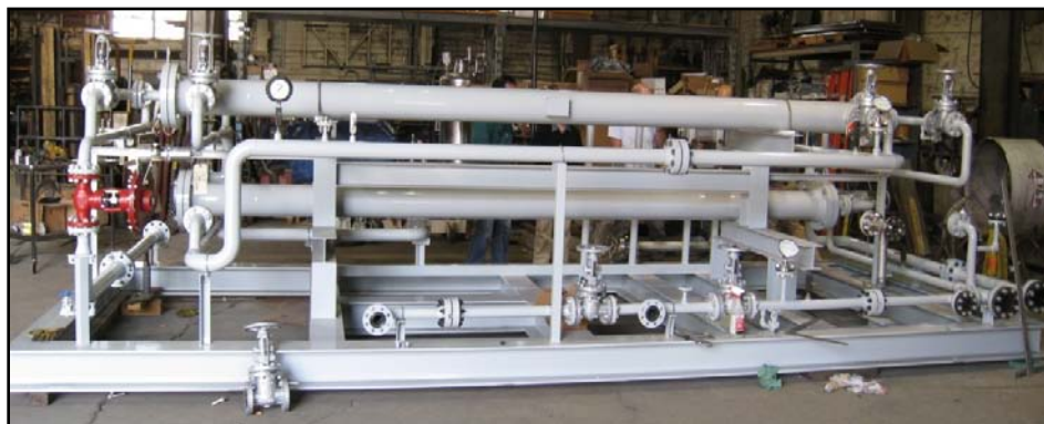
Figure 5: Membrane Skid Used for Six-Month Pilot-Scale Slipstream Test Conducted at APS's Cholla Power Plant
