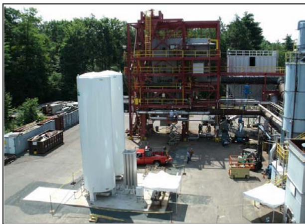
Figure 2: Photo of BSF with Oxy Modifications
