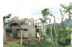
High wind damage
