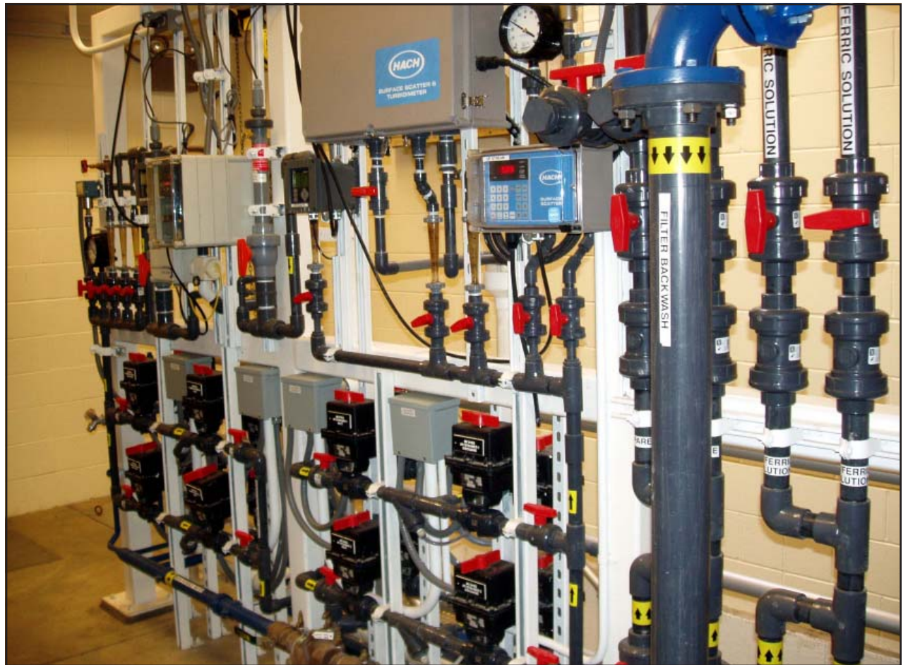
Part of a coagulation/filtration treatment system in Billings, Montana.
