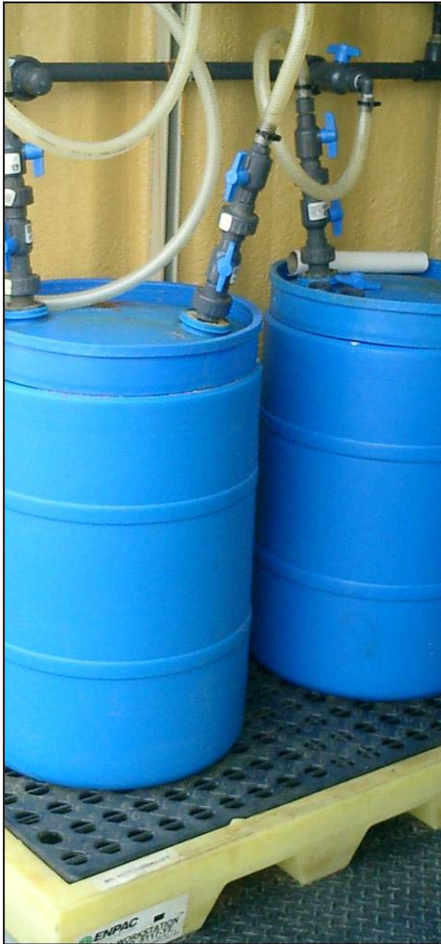
Adsorptive media treatment system for ion exchange waste brine.
