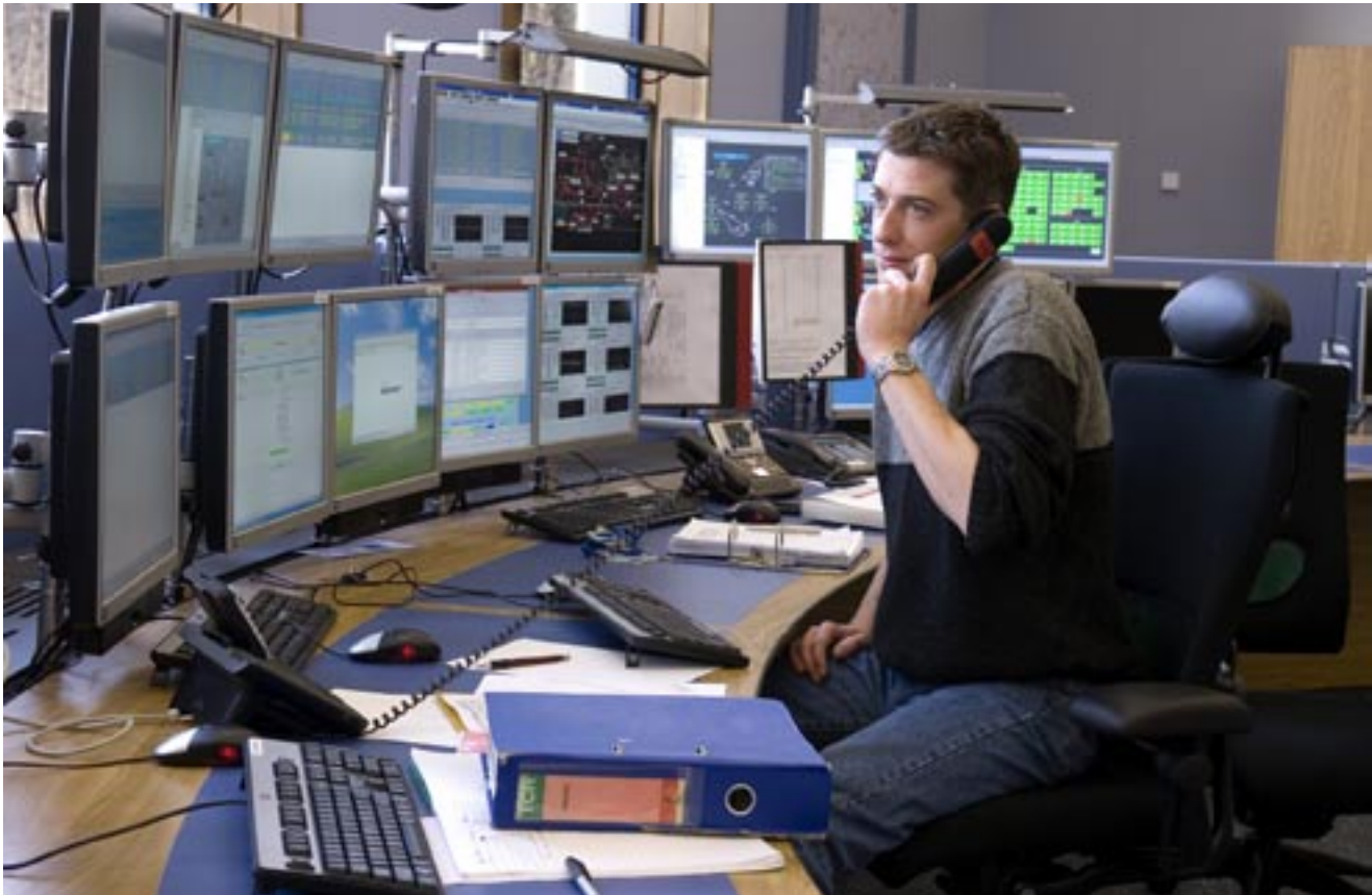
The control center at CERN—the European Organization for Nuclear Research, a frequent user of the GLORIAD network—combines all control rooms for the accelerators, the cryogenic system, and the technical infrastructure. ©CERN
