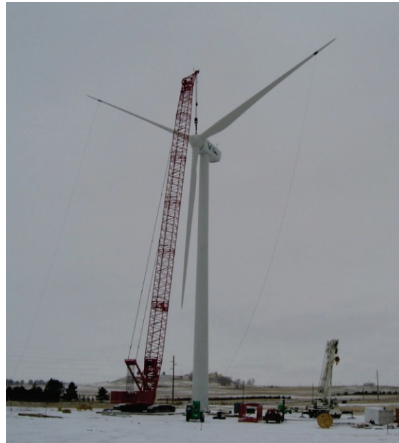
Figure 2-2. Installation of Rotor Blades on a 2.0-MW Turbine at Warren Air Force Base, Wyoming (total height = 367 ft)
