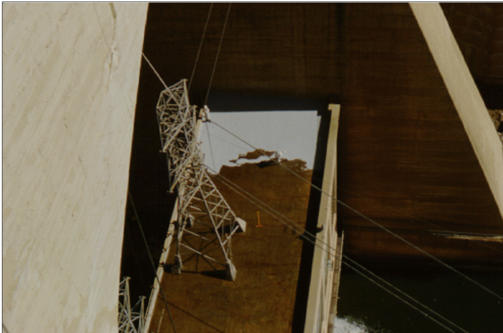
Figure 61.—The thin PC overlay system can be applied very quickly. Two workmen completed application to this powerplant roof in 2 days.
