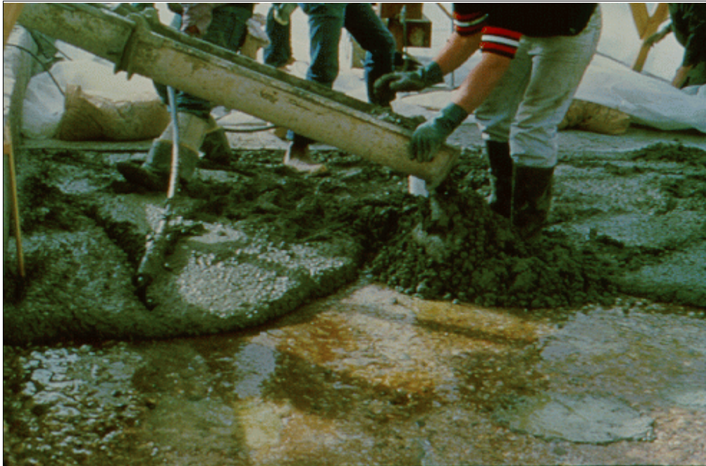
Figure 56.—The placement techniques for epoxy-bonded concrete are essentially the same as for conventional concrete.
