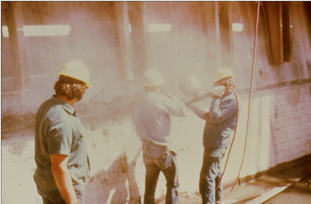
Figure 40.—A small size pneumatic gun can be used to apply portland cement mortar. Regular shotcreting equipment would be too large for this application.
