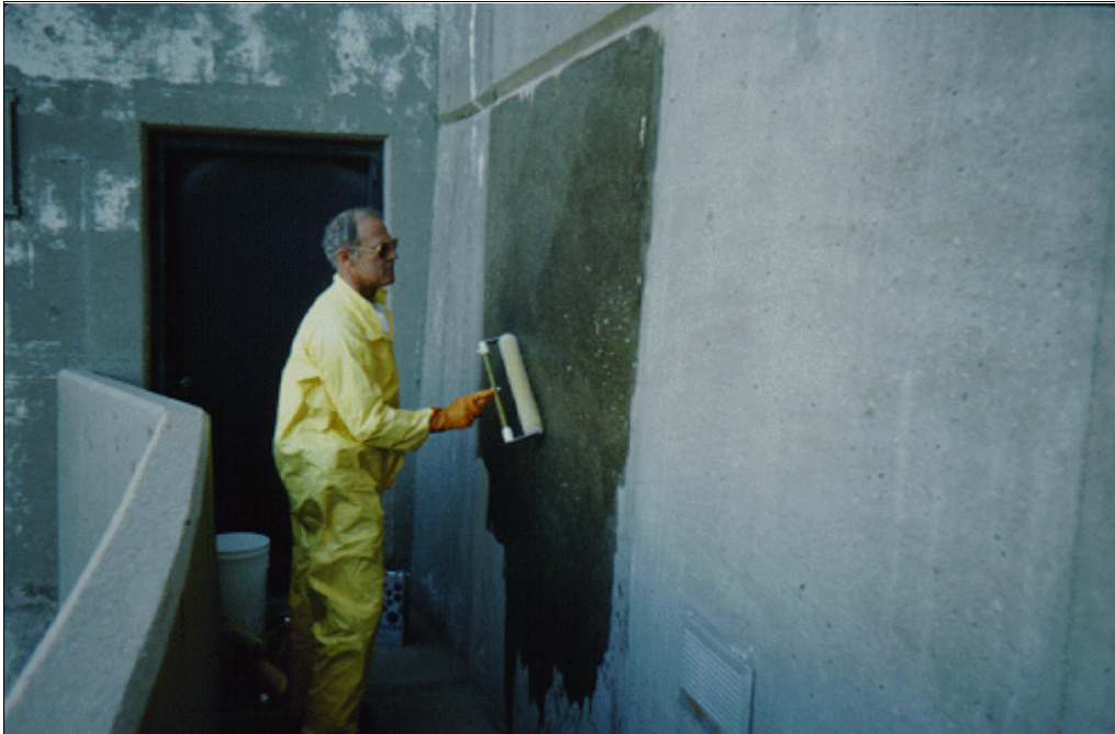
Figure 72.—A paint roller application of siloxane sealing compound to the downstream face of Nambé Falls Dam, near Santa Fe, New Mexico.
