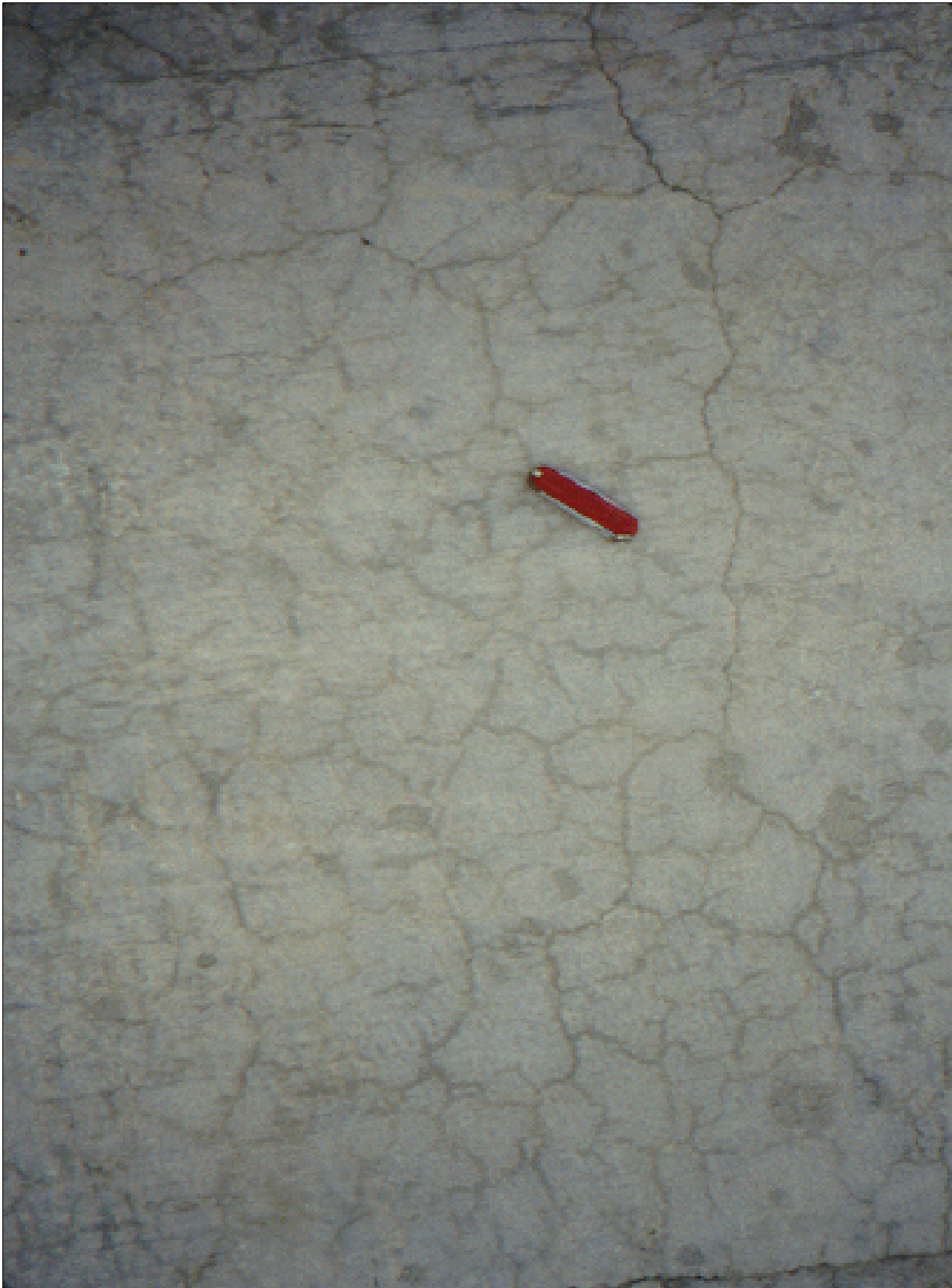
Figure 32.—Typical appearance of drying shrinkage cracking.
