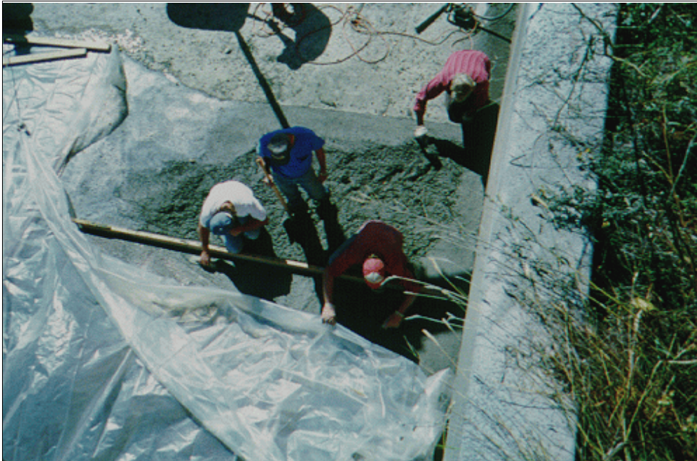
Figure 71.—Curing compound and polyethylene sheeting should be applied to cure silica fumeconcrete as soon as finishing is completed if drying shrinkage cracking is to be prevented.
