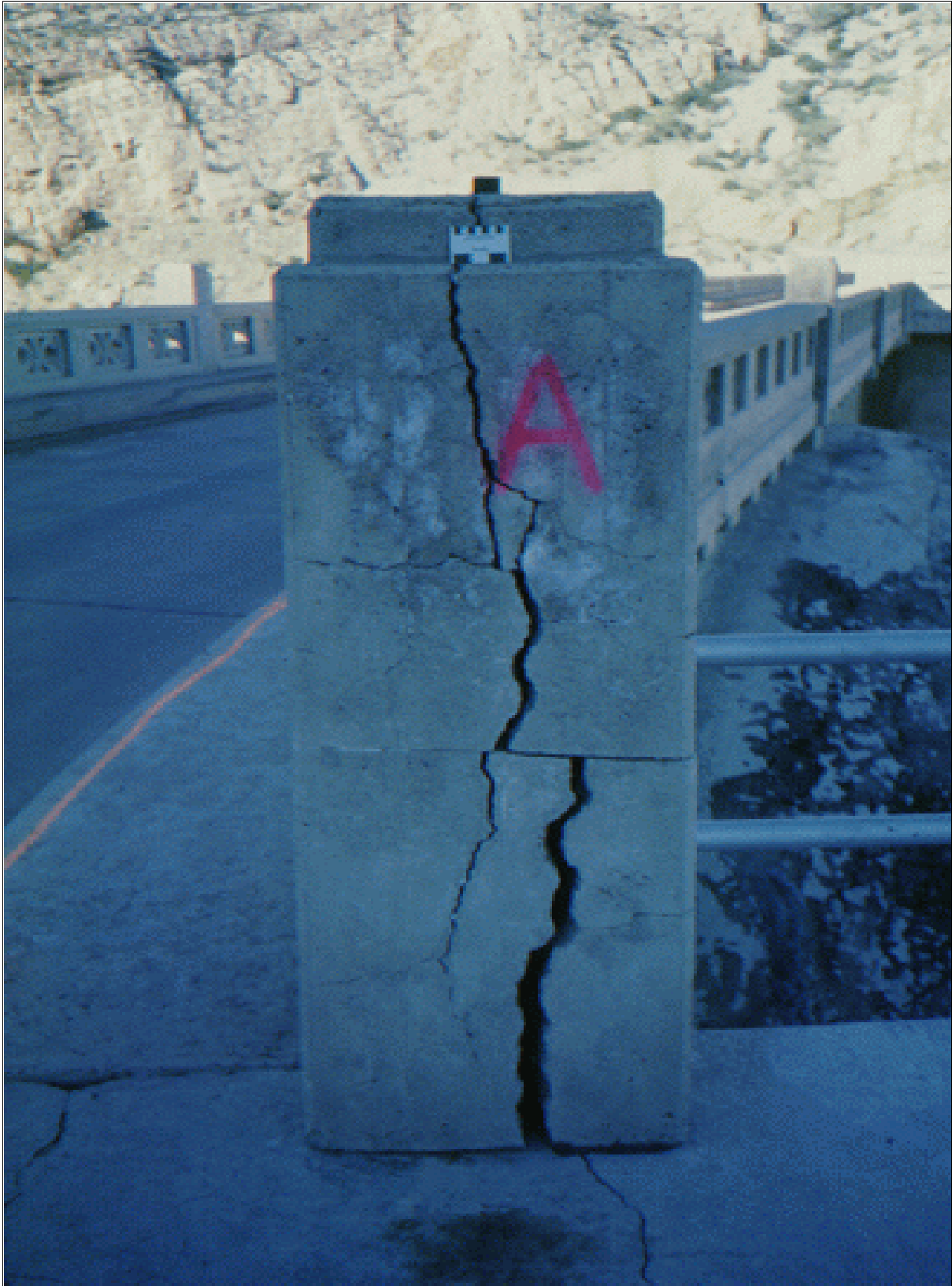
Figure 19.—Severe cracking caused by alkali-aggregate reaction.
