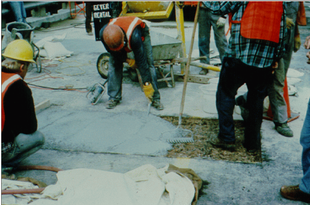
Figure 58.—Small stinger vibrators can be used to consolidate shallow depths of polymer concrete.
