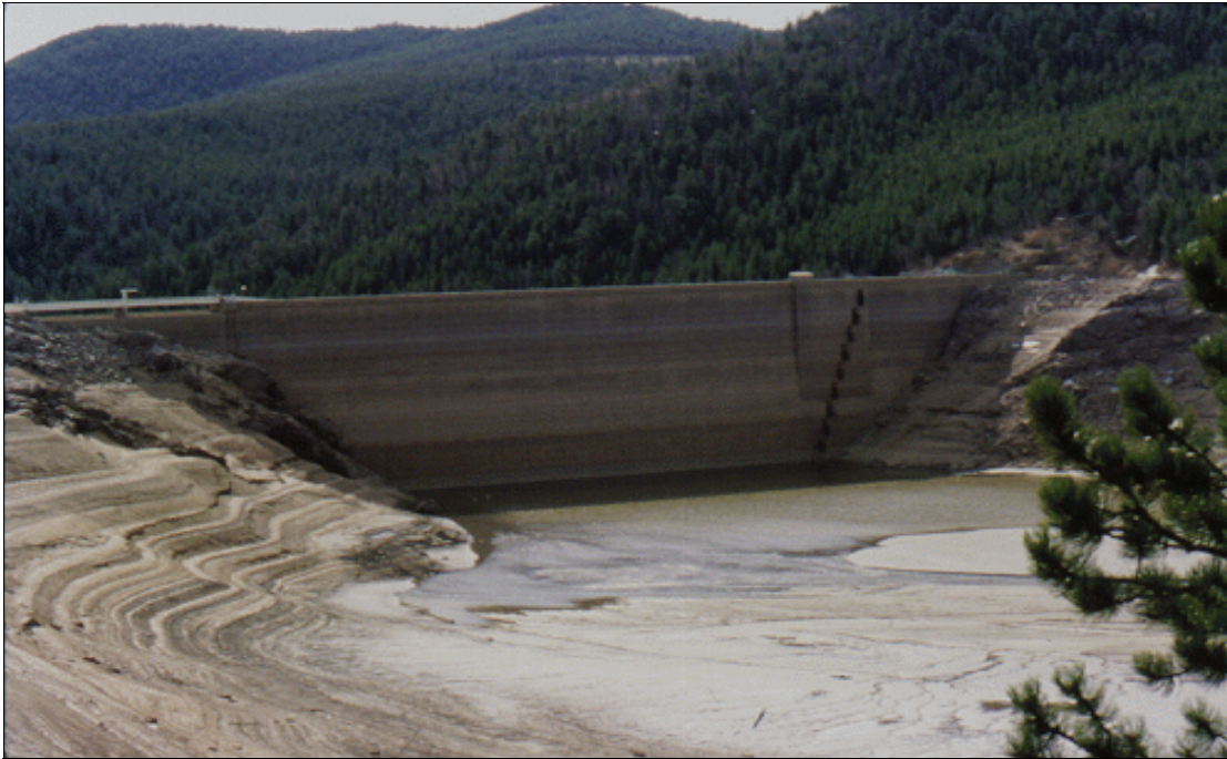
Figure 42.—The downstream face of Barker Dam, near Boulder, Colorado, was resurfaced with prepacked aggregate.
