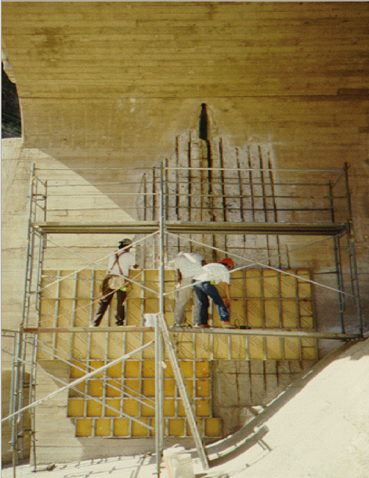
Figure 55.—If forms are required for epoxy-bonded concrete repairs, they should be installed at least once prior to application of the epoxy bond coat to ensure that they fit as planned and that they can be installed and filled before the bond coat hardens.
