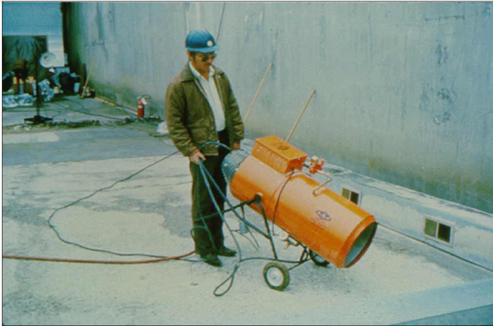
Figure 49.—A gas-fired forced air heater is being used to heat concrete prior to application of epoxy mortar.
