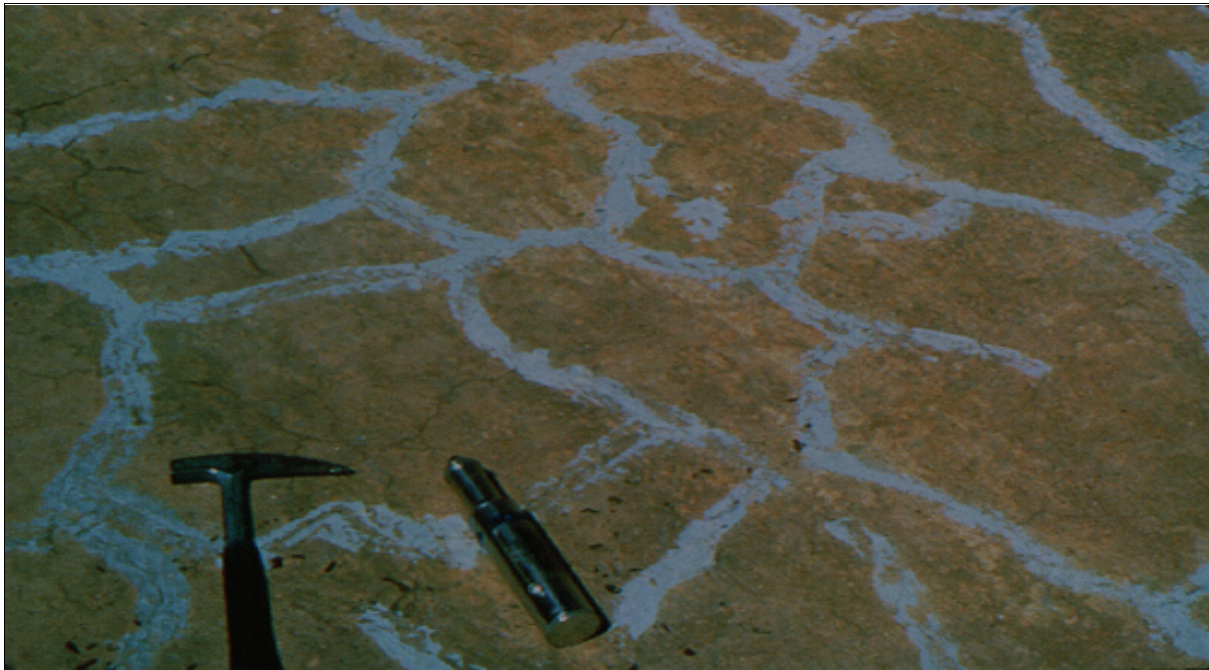
Figure 34.—Inadequate crack repair techniques often result in poor appearance upon completion.
