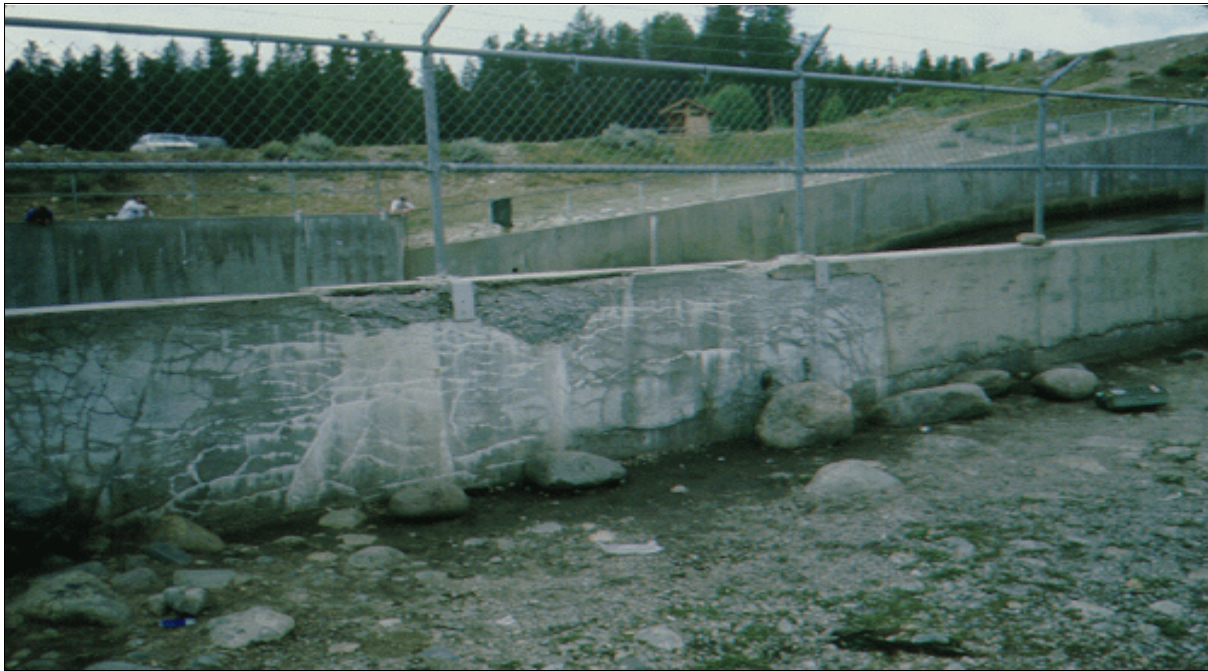
Figure 22.—D-cracking type of freezing and thawing deterioration.
