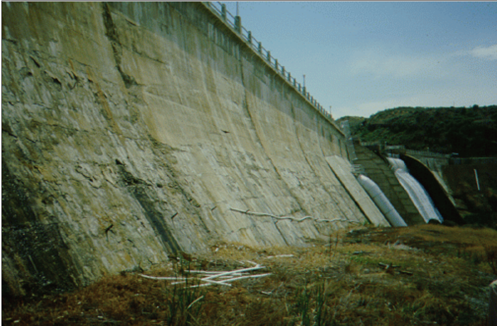
Figure 3.—Freezing and thawing deterioration to the downstream face of this dam does not require repair for safe operation of the structure.
