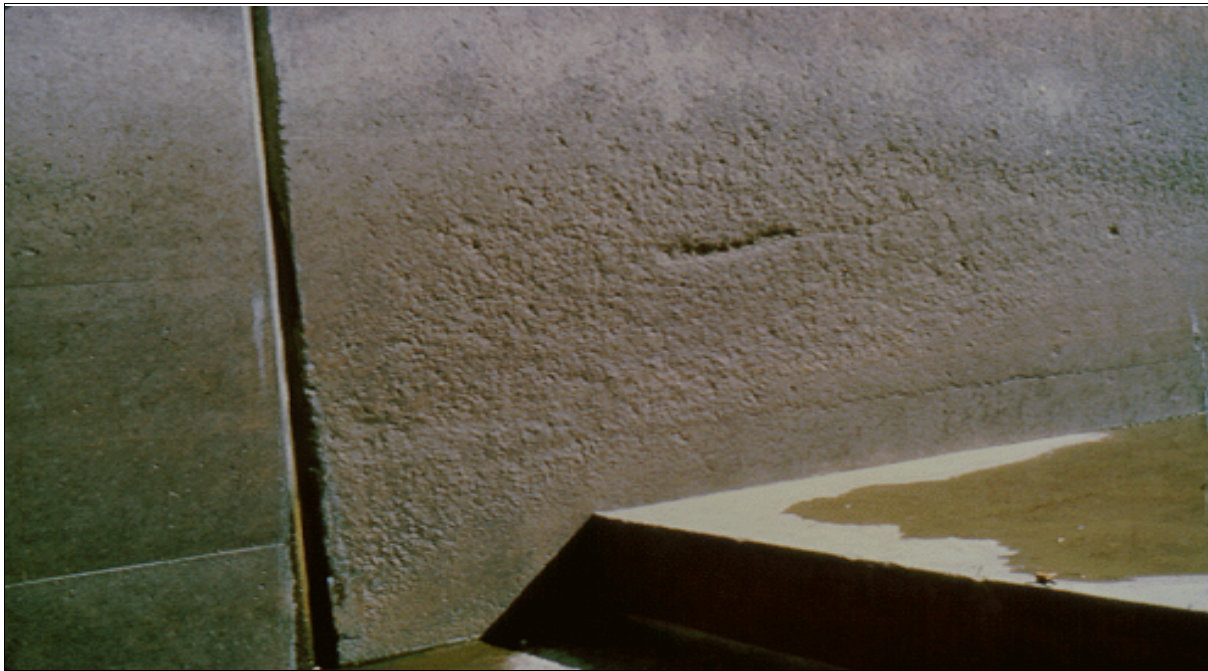
Figure 25.—Early stages of abrasion-erosion damage.
