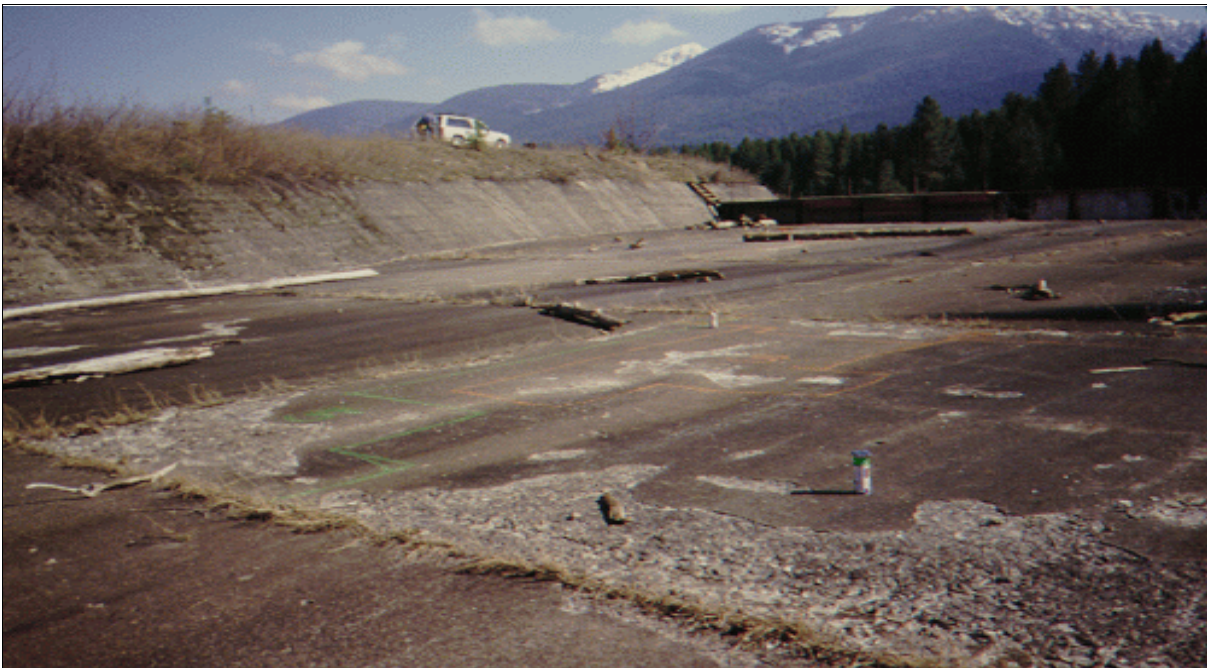
Figure 21.—Freezing and thawing deterioration on spillway concrete.
