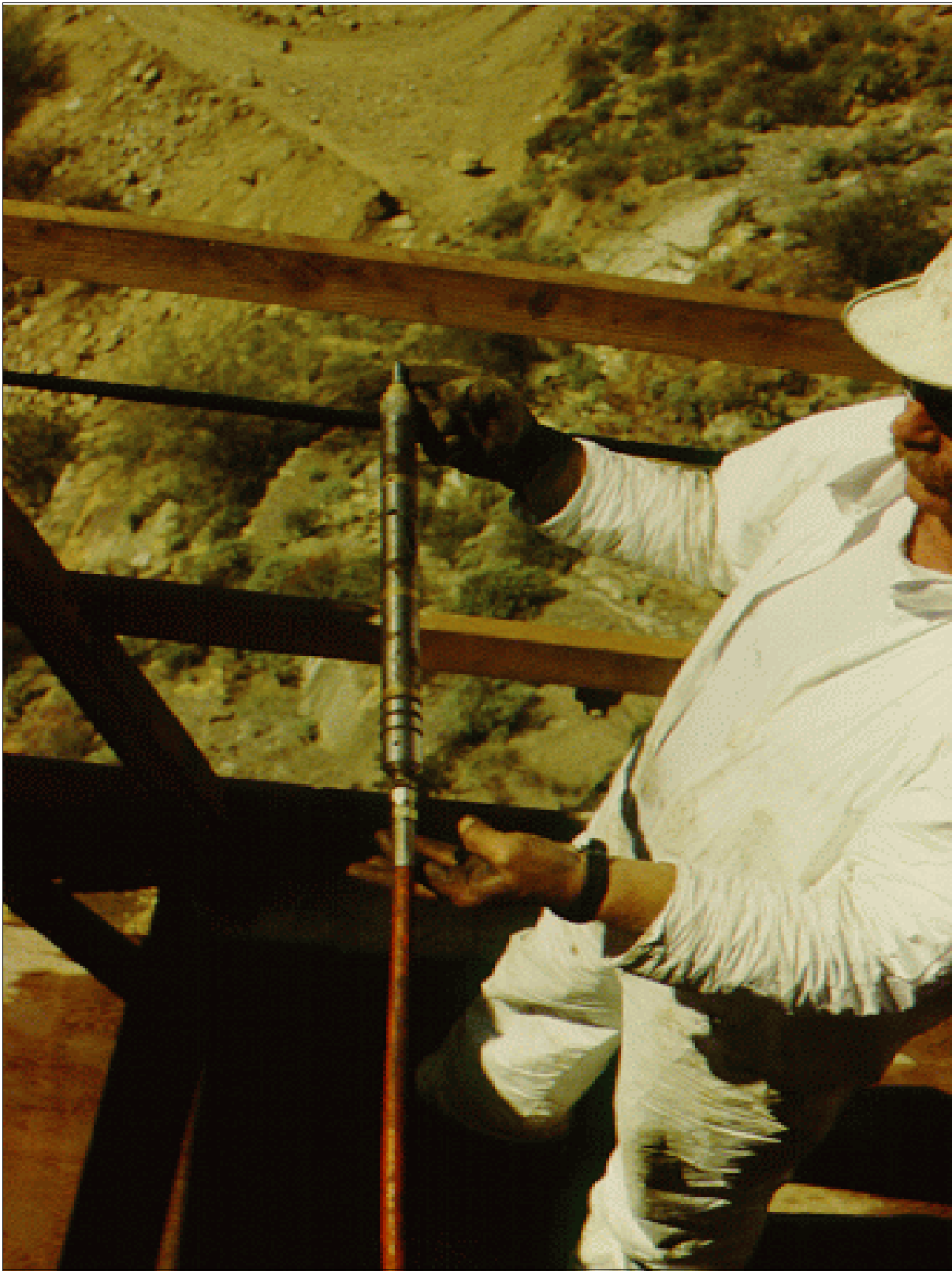
Figure 67.—A proprietary downhole packer allows separation of the resin components until they reach the downhole point of injection.
