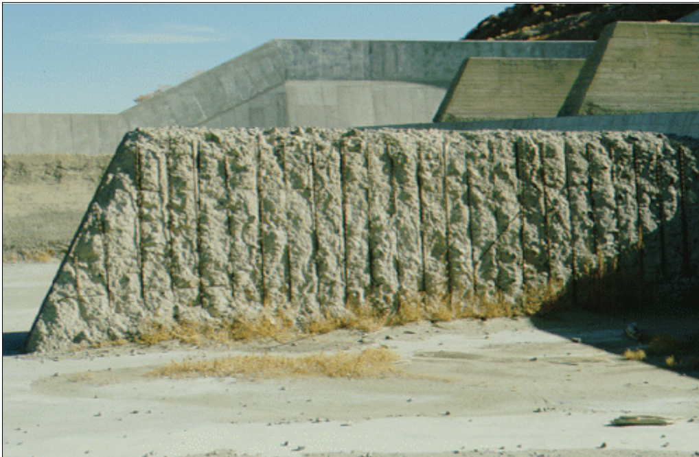
Figure 4.—This freezing and thawing deterioration should have been repaired before it advanced to the point that wall replacement or removal is the only option.
