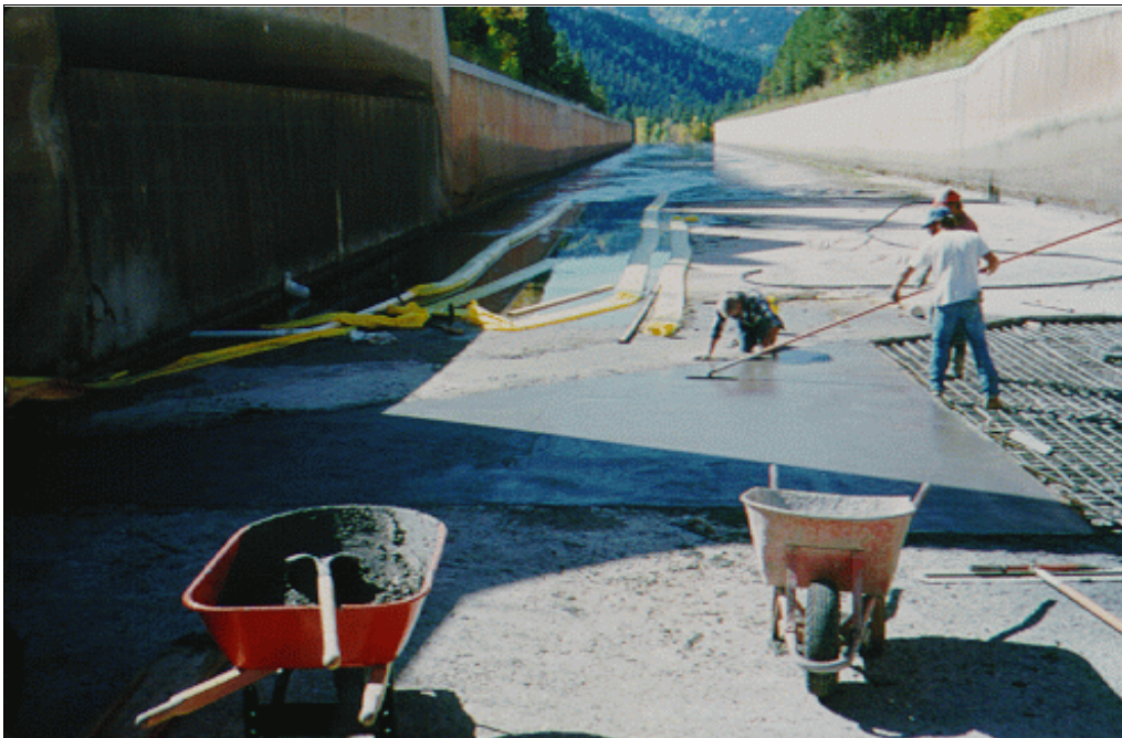
Figure 70.—Using a bull float on a silica fume repair. Finishing must be done immediately after screeding.
