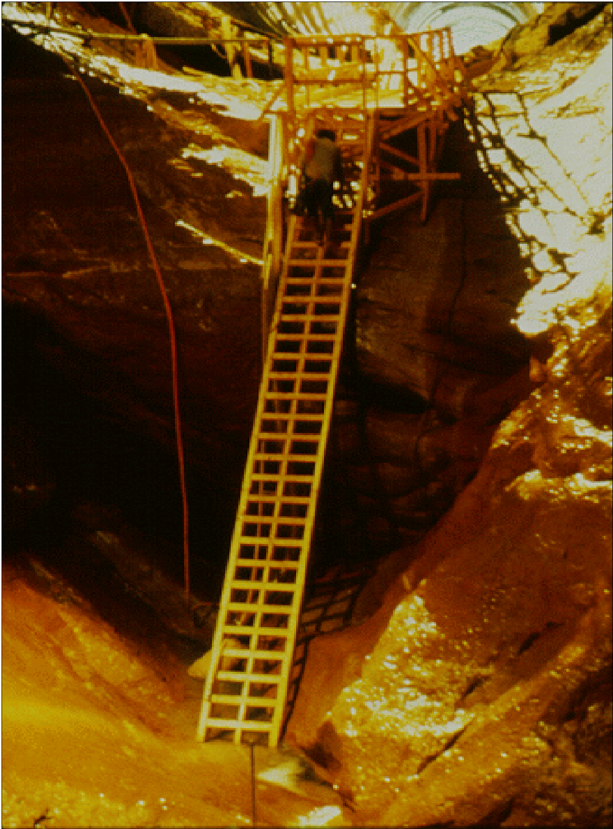
Figure 28.—Extensive cavitation damage to Glen Canyon Dam.
