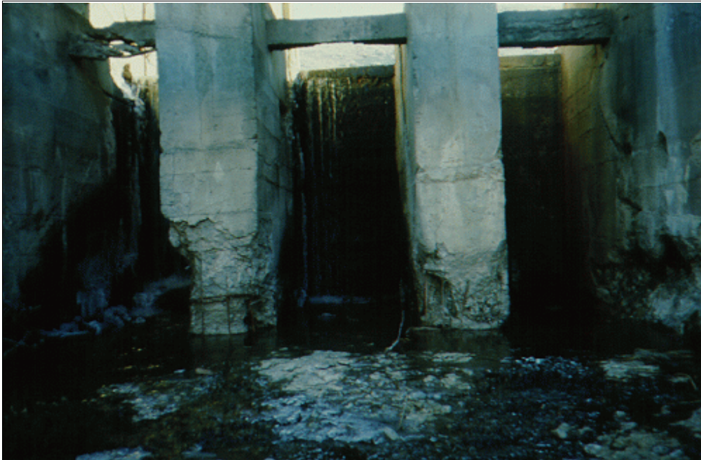
Figure 1.—Lack of maintenance has resulted in near loss of this irrigation structure.
