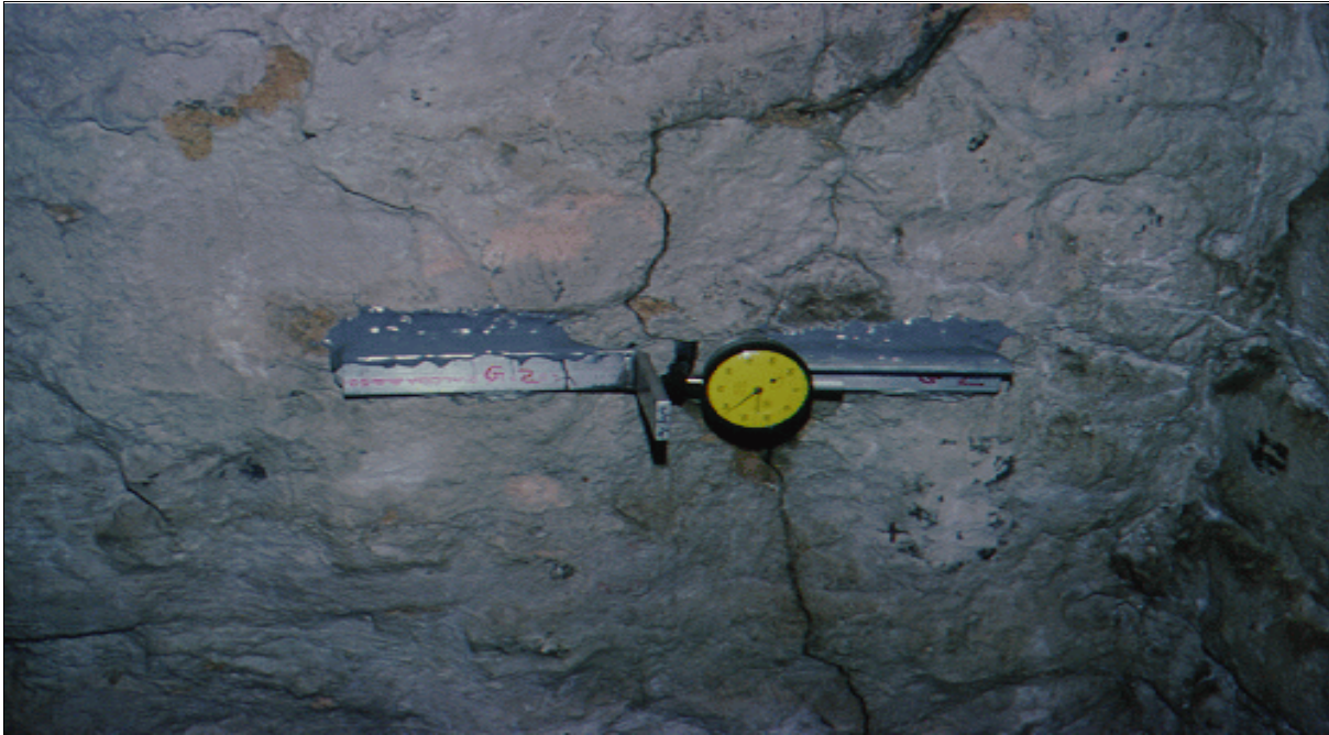
Figure 36.—Crack gage installed across a crack will allow determination of progressive widening or movement of the crack. It may be necessary to monitor such gages for periods up to a year to predict future crack behavior.
