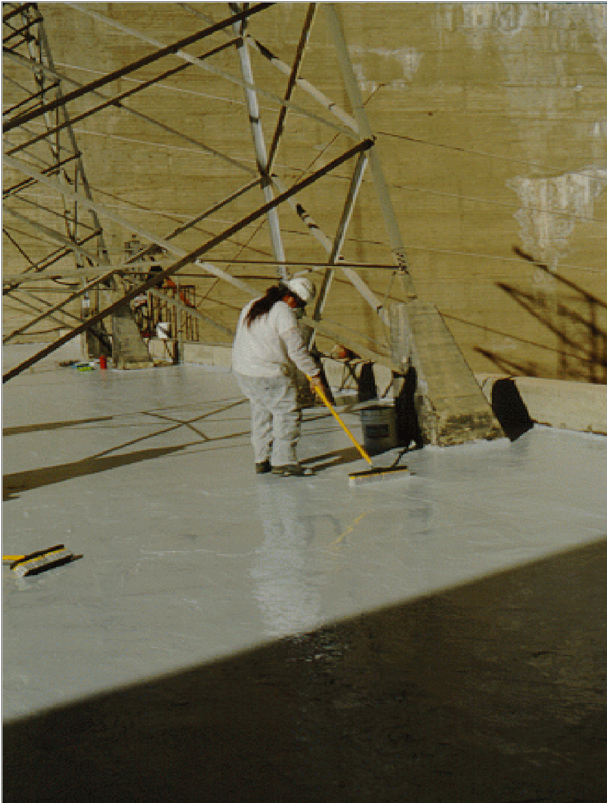
Figure 60.—The thin PC overlay system may be applied with push brooms, squeegees, or heavy industrial grade paint rollers.
