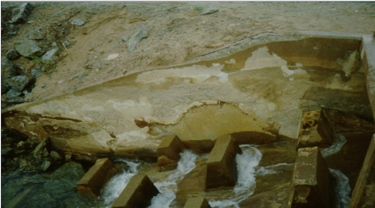
Figure 29.—Concrete damage caused by chloride-induced corrosion of reinforcing steel. The waters contained within this flume had high chloride content.
