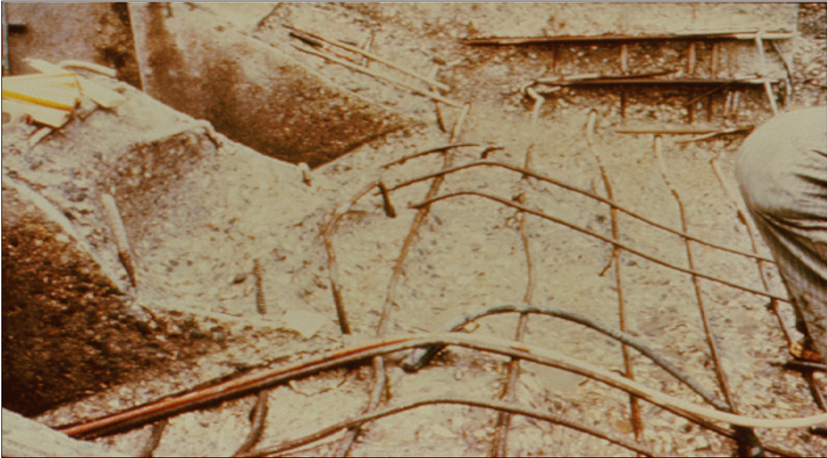
Figure 23.—Abrasion-erosion damage in a concrete stilling basin.
