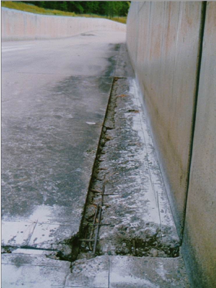
Figure 7.—This concrete damage was found to be a serious threat to the structural integrity of this spillway.
