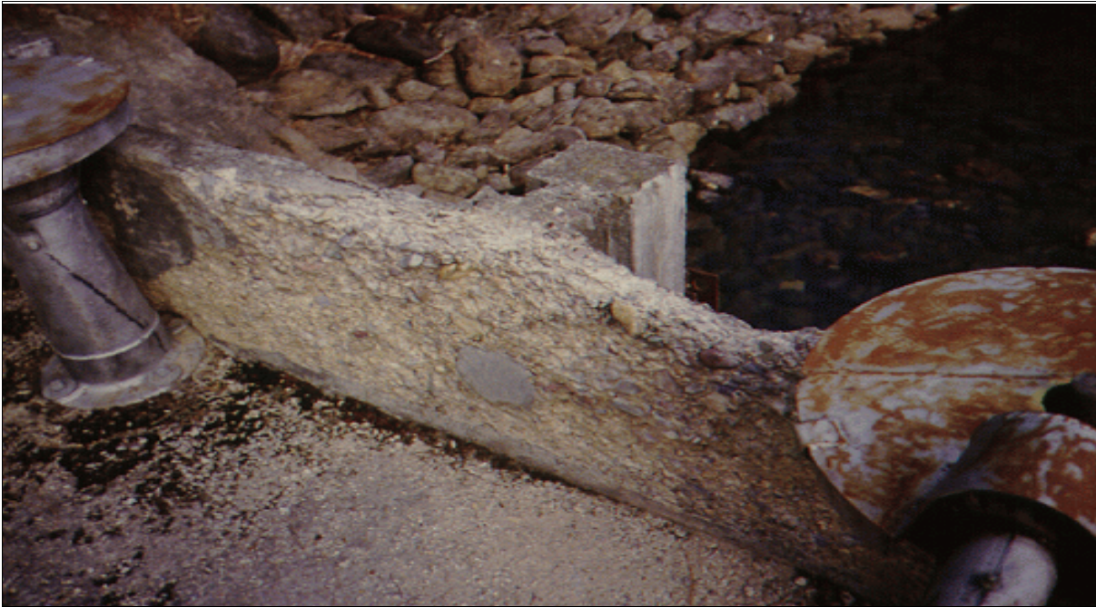
Figure 20.—Freezing and thawing deterioration on small irrigation gate structure.
