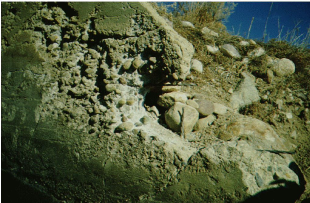
Figure 2.—Deferred maintenance has allowed freezing and thawing deterioration to seriously damage this structure.
