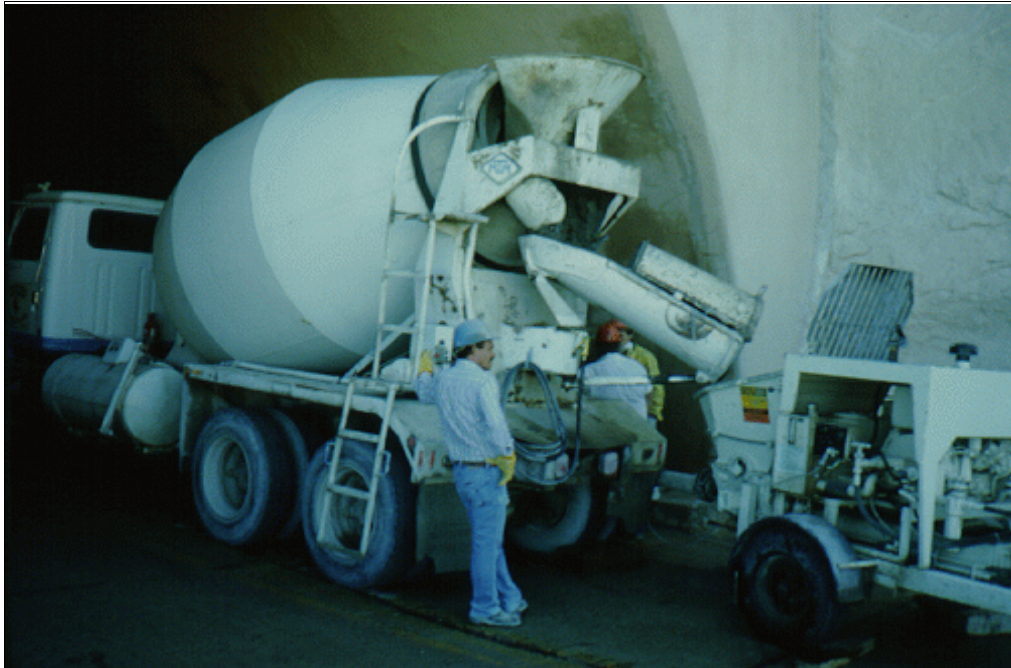
Figure 45.—Wet mix shotcrete equipment. The premixed shotcrete is delivered to the shotcrete pump by a transit truck.
