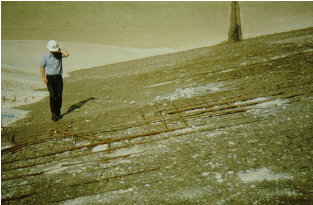
Figure 6.—Spillway damage requiring repairs at some future date.
