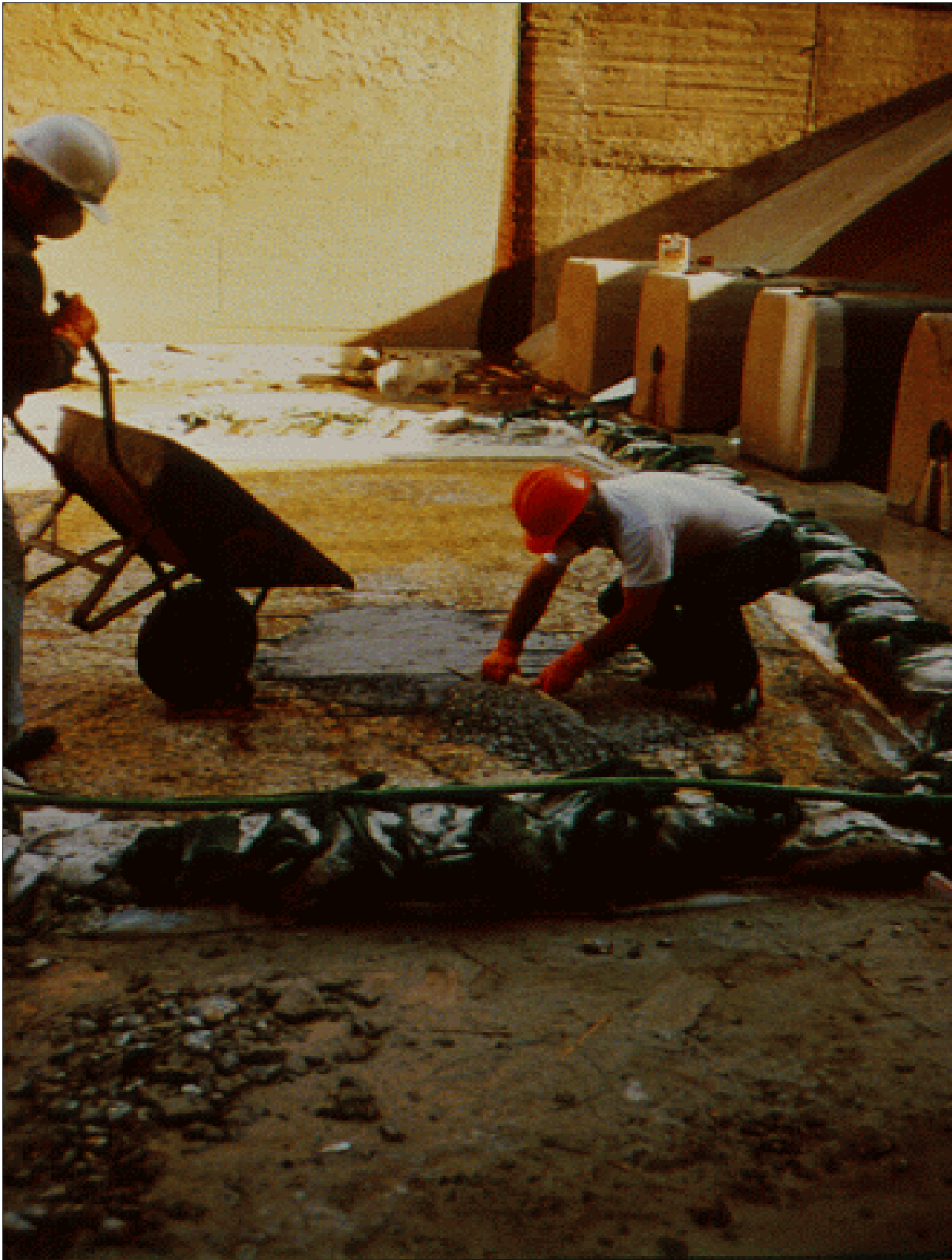
Figure 57.—Placing polymer concrete in a repair area. Sandbags and polyethylene sheeting were used to prevent water from entering the repair area.
