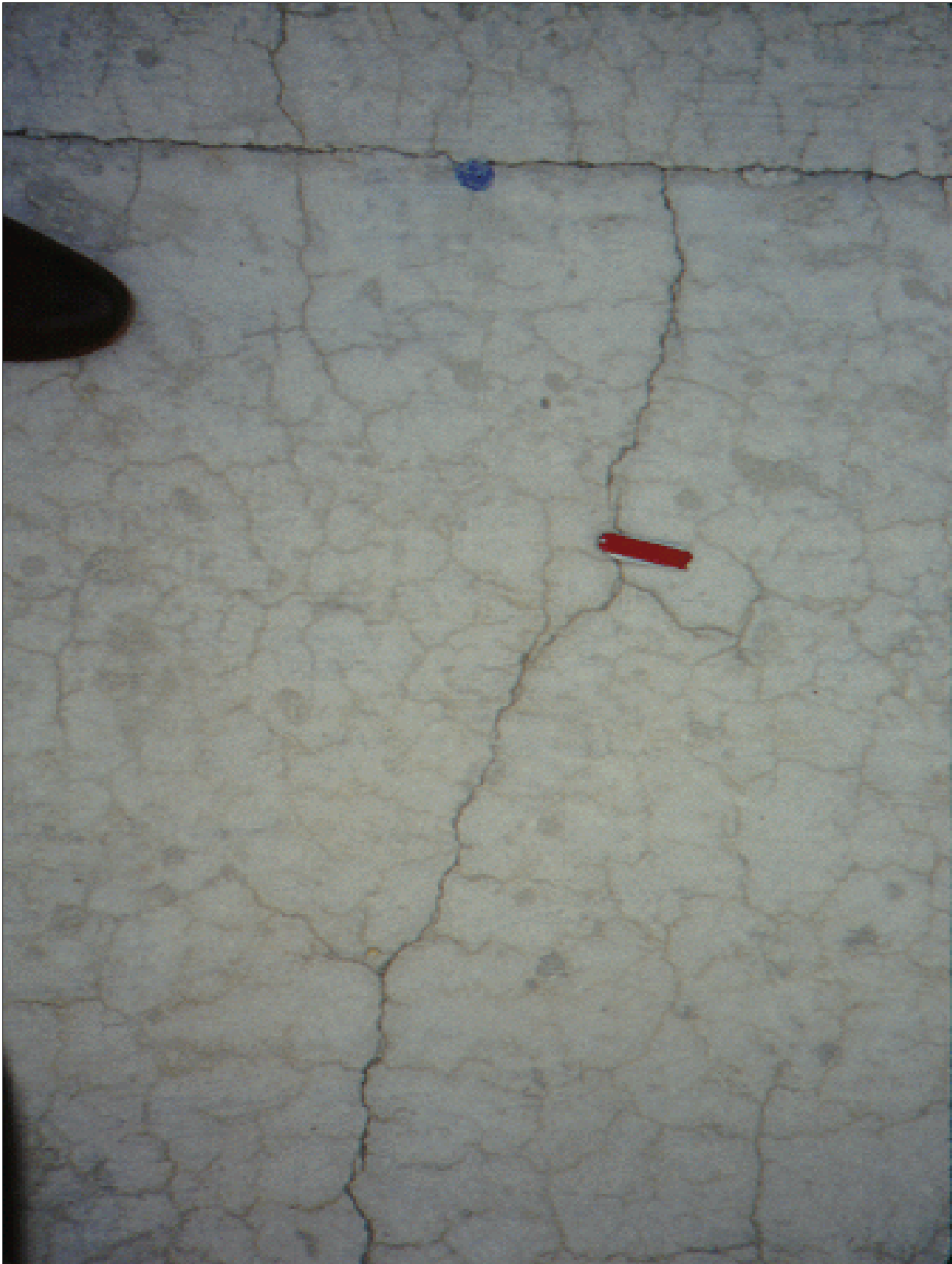
Figure 37.—A large reflective crack has formed in a concrete overlay which also exhibits circular drying shrinkage cracking.
