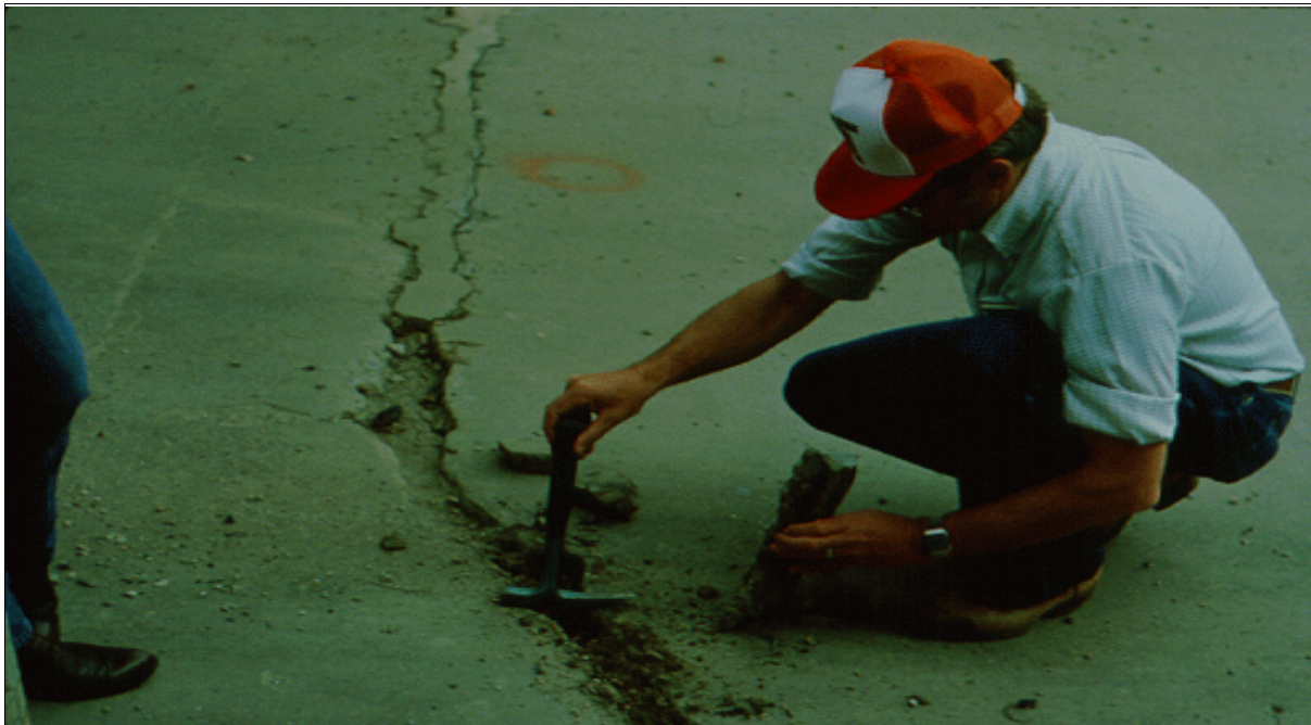
Figure 35.—Improper crack repair techniques often result in short service life.
