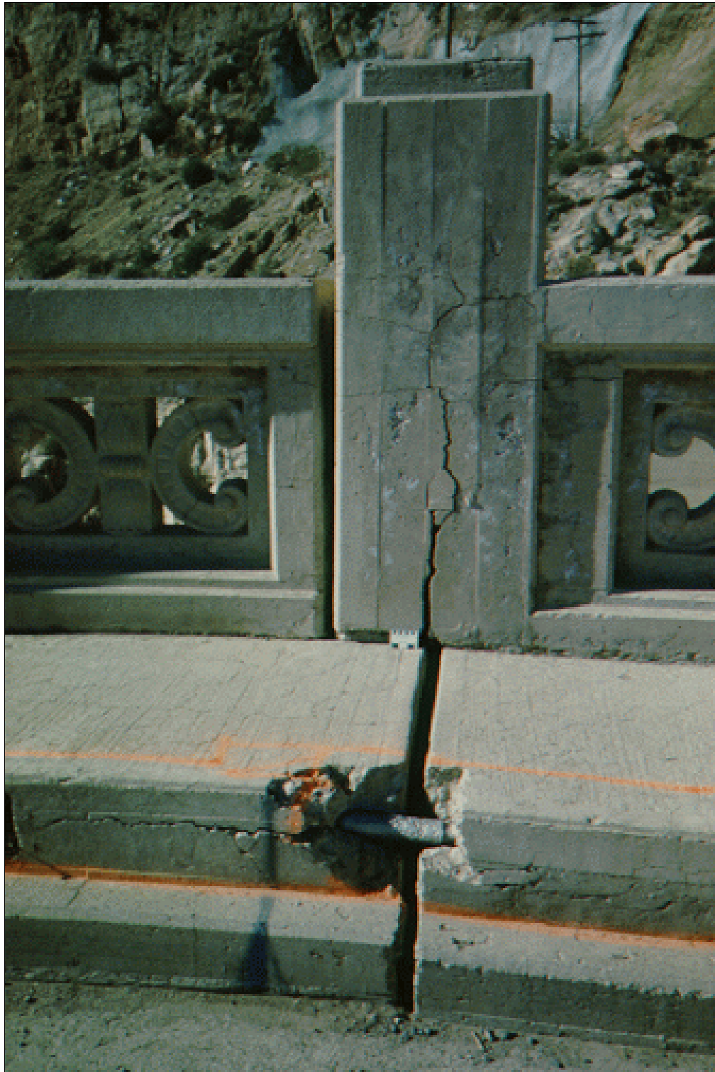
Figure 38.—Multiple causes of damage are apparent in this photograph. Poor design or construction practices placed the electrical conduit too near the surface. A combination of freezing and thawing deterioration and alkali-aggregate reaction is responsible for the cracking and surface spalling on the parapet wall.
