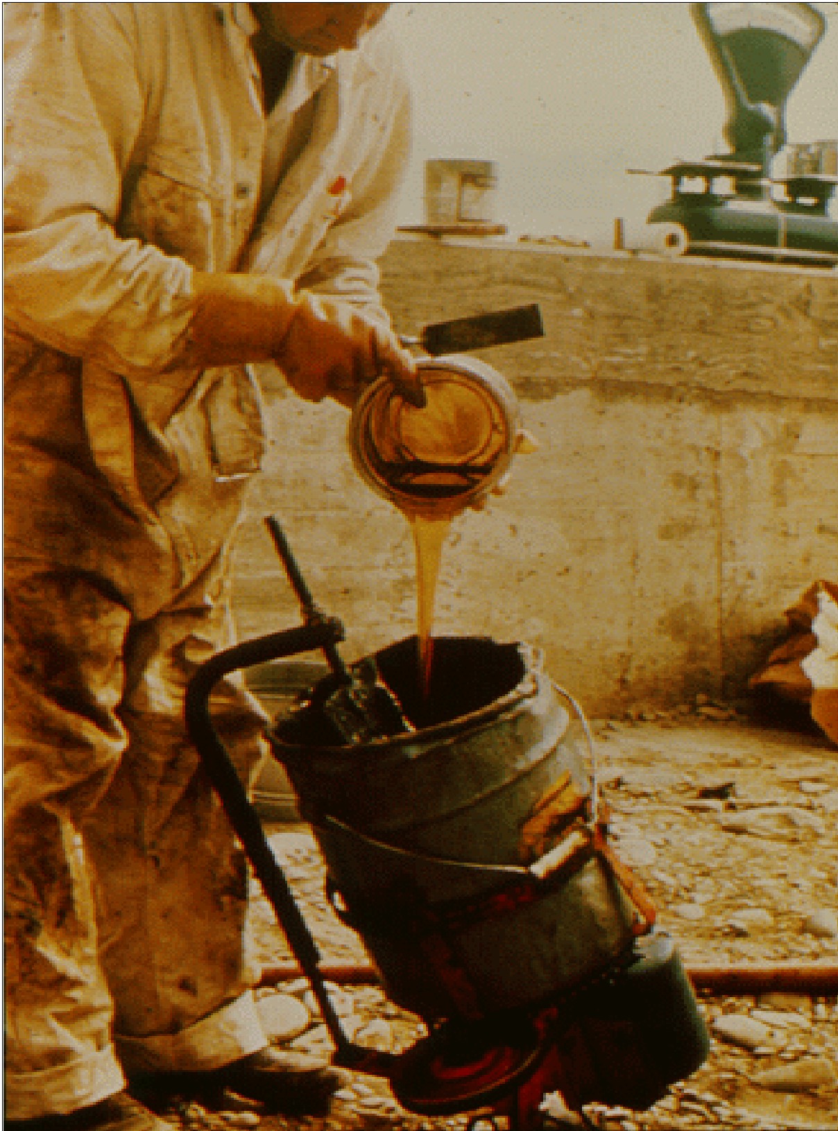
Figure 51.—A bucket mixer can be used to mix epoxy mortar for small repair areas.
