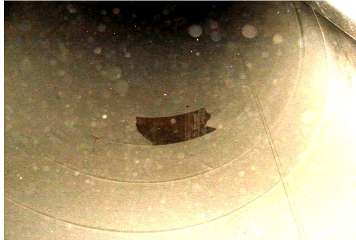
Figure 2.2-4. Inside of stack 1 approximately 30 ft from the bottom. The dark brown area exposes the liner where a 4ft x 8ft section of buildup had fallen off.
