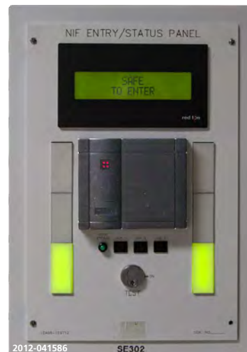
Figure 4-4: SIS entry panel and access control system (ACS) badge reader used to control facility access. ACS is used by operations staff to tell who is where in the facility.
