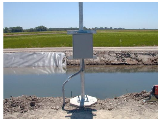
FIGURE A-3 Installed SonTek Control Panels
