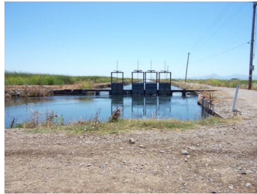
FIGURE A-7 Banion Check Structure on Belding Lateral Showing High Water Levels
