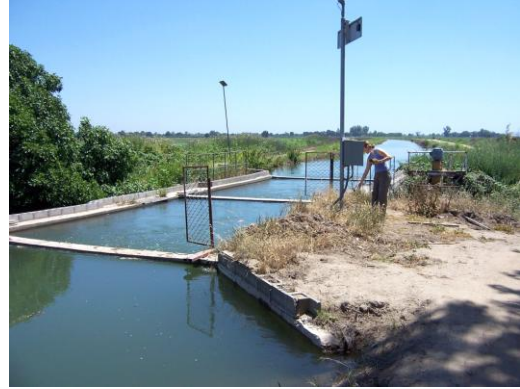
FIGURE A-6 Nugent Flume on Traynor Lateral at Near-Peak Flow Condition Showing High Water Levels
