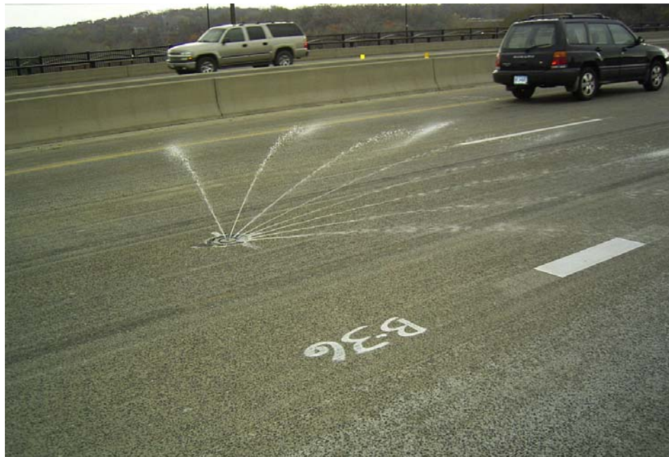
FIGURE 45 Anti-icing system on a bridge.
