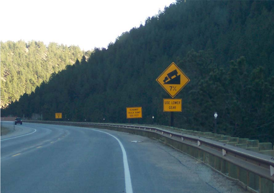
FIGURE 95 Guardrail on the outside of a horizontal curve.
