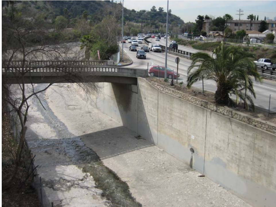
FIGURE 117 The Arroyo Seco Channel runs adjacent to the Parkway, constraining its width on one side.
