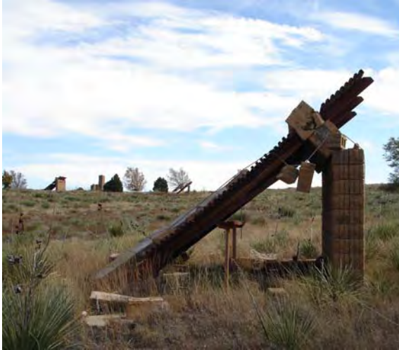
Unsafe Picnic Structure
