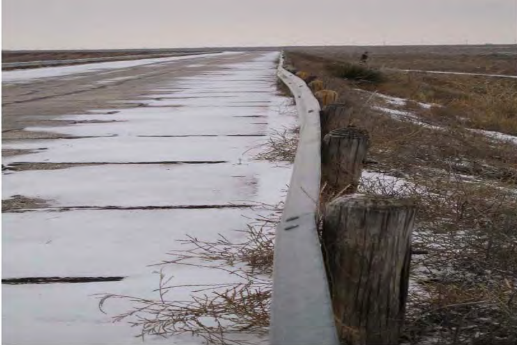
Photograph 4 – Current Condition of the Road and Guardrail Across Top of Dam
