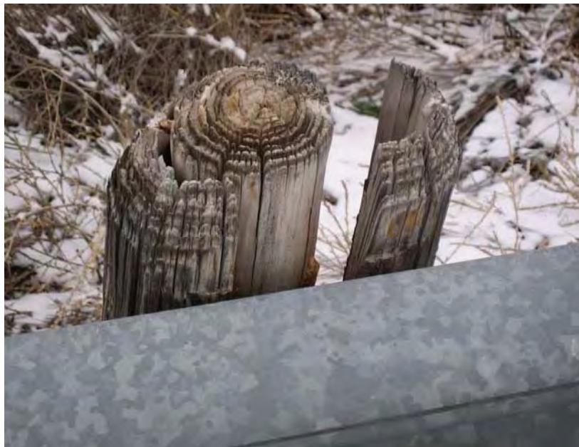
Photograph 5 – Present Condition of Some Guardrail Posts
