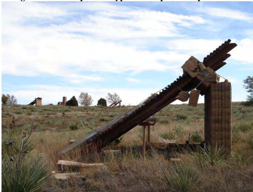
Figure 2-4 Example of a Typical Collapsed Campsite Shelter
