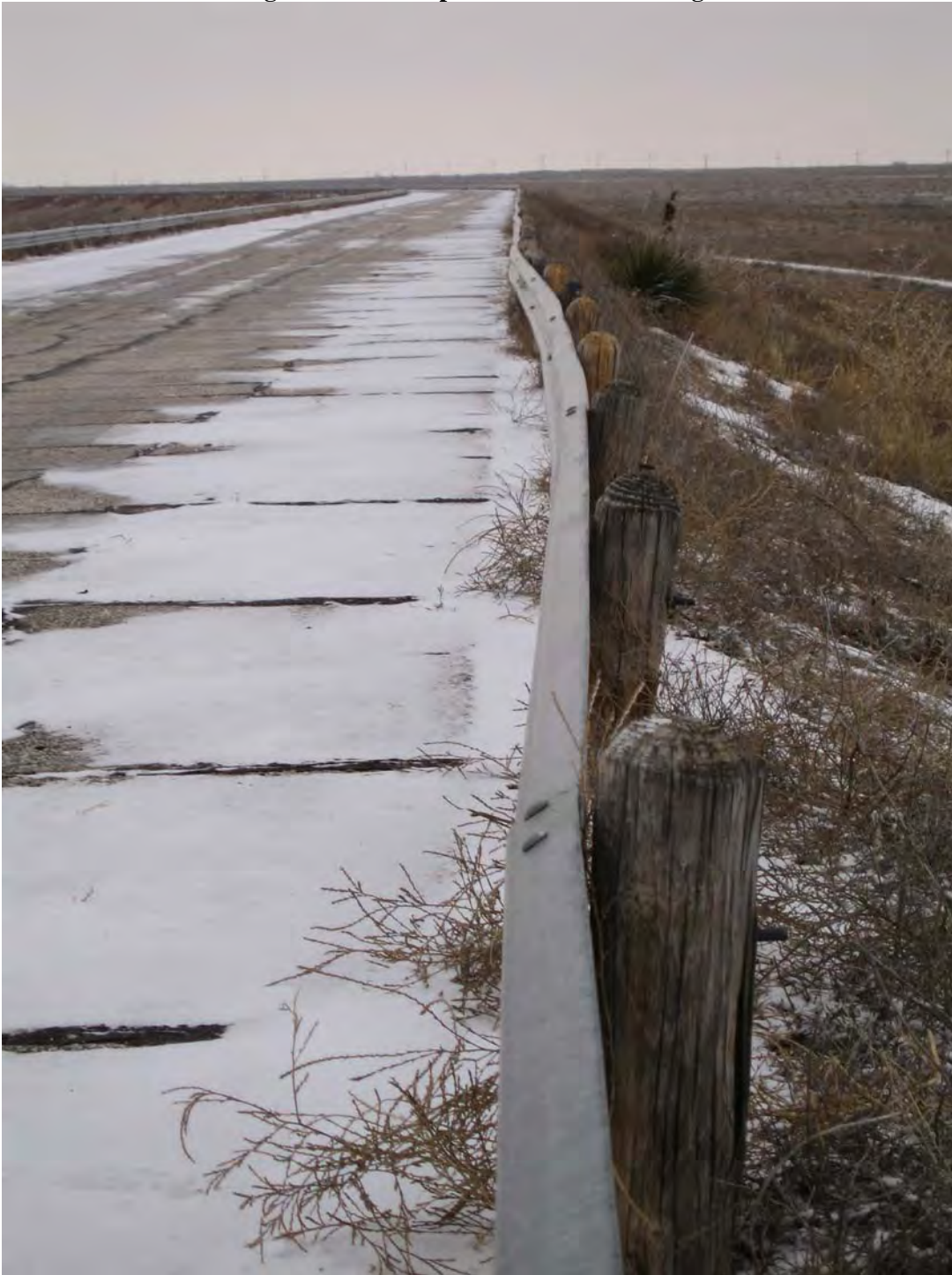
Figure 1-3 Example of Guardrail Damage
