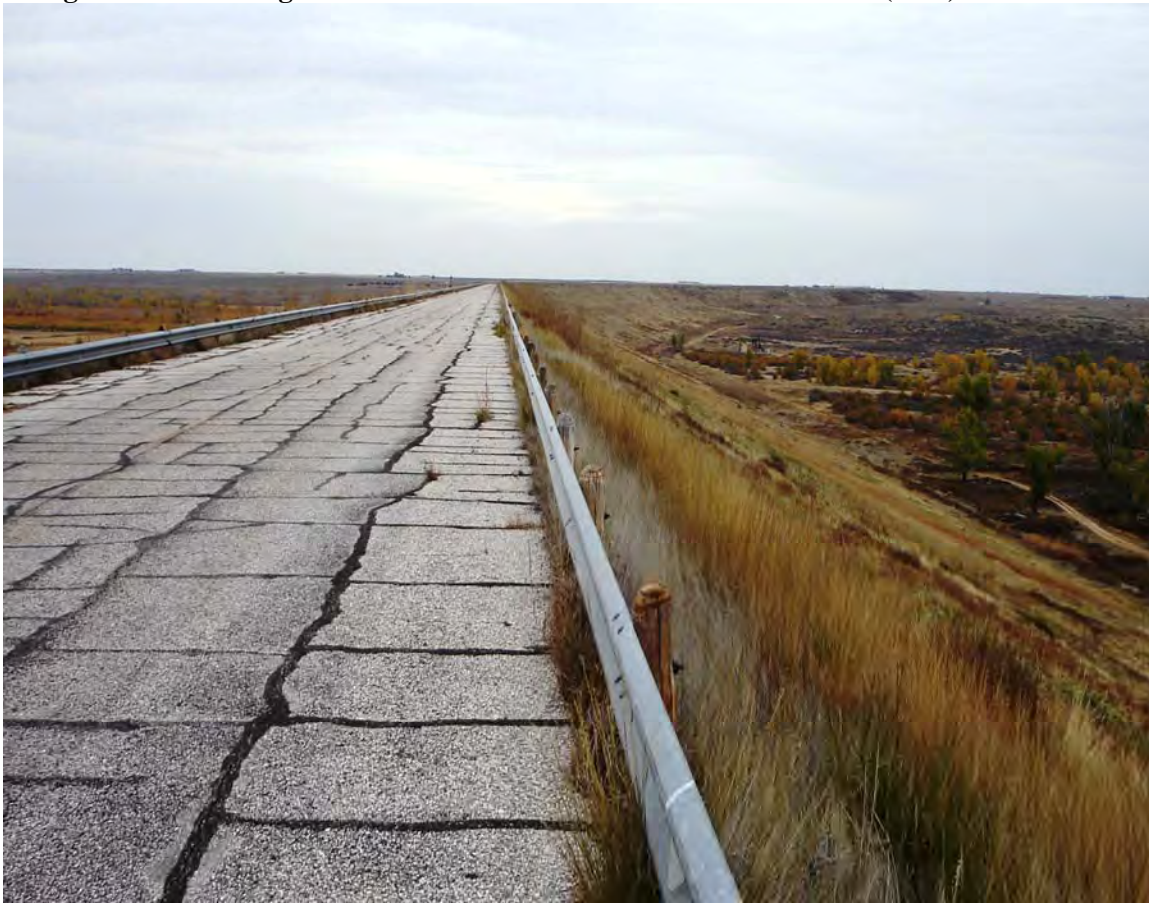
Figure 1-2 Looking North at Road and Guardrail on Downstream (East) Side of Dam
