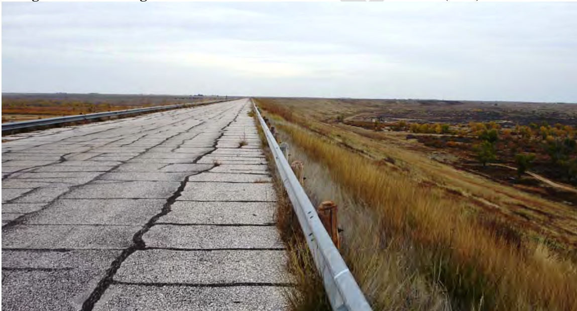
Figure 1-2 Looking North at Road and Guardrail on Downstream (East) Side of Dam
