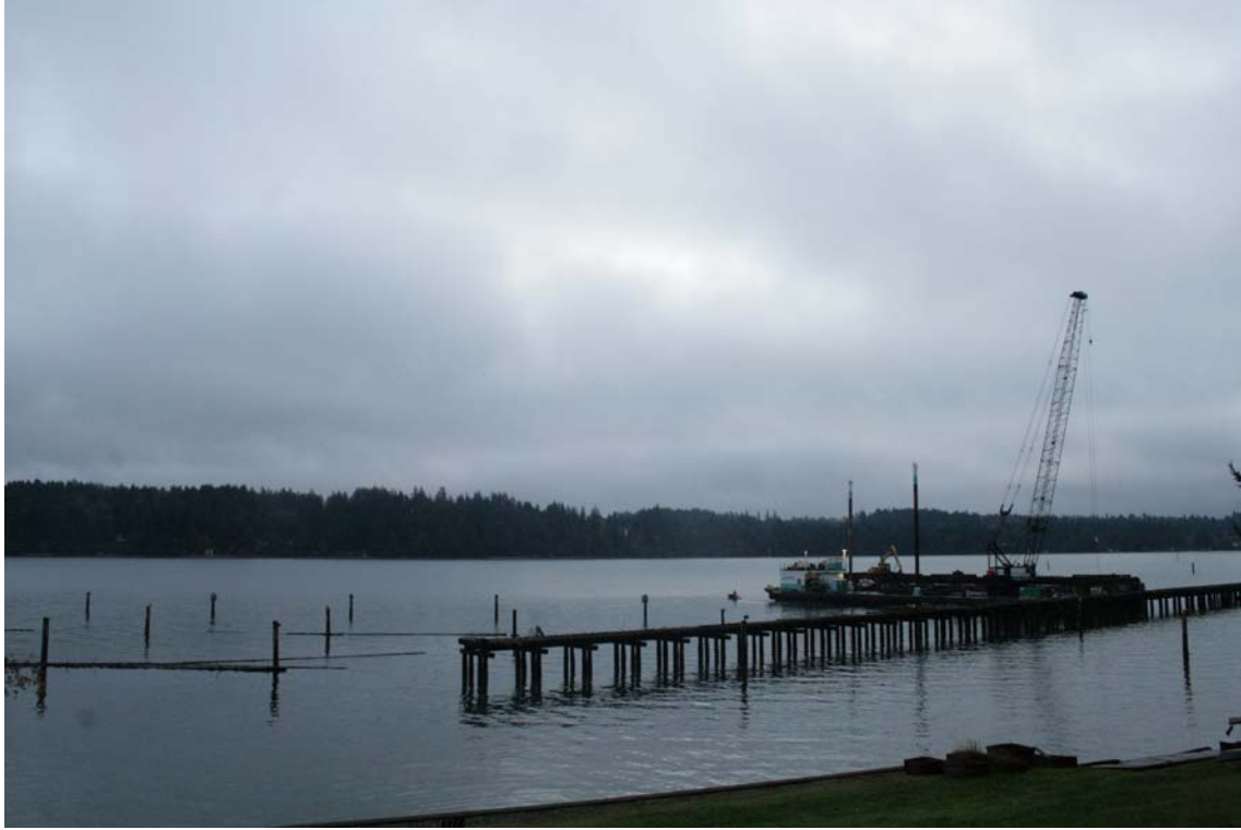
Figure 2. View of barge and crane working adjacent to North Seal Haul-out from PSO observation area.
