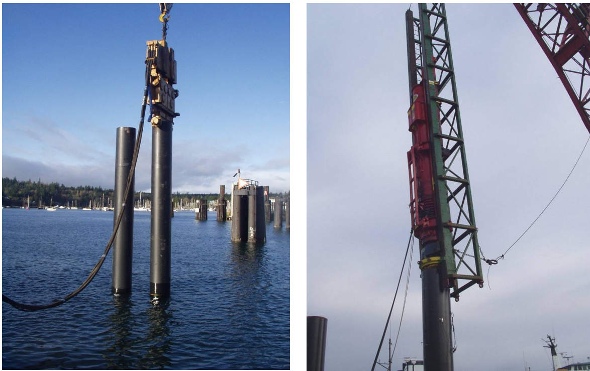
Figure 1-8. Impact Hammer Driving a Pile (Left), Vibratory Hammer Driving a Pile (Right)
