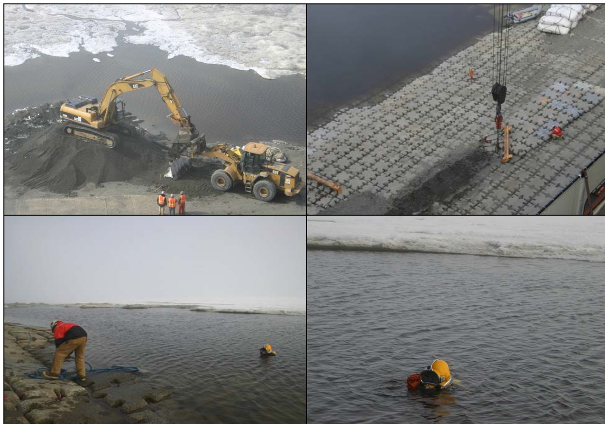
FIGURE 1.7. Block system and fabric repair (above left and right) and diver repair work (bottom left and right) at Northstar Island in 2009.
