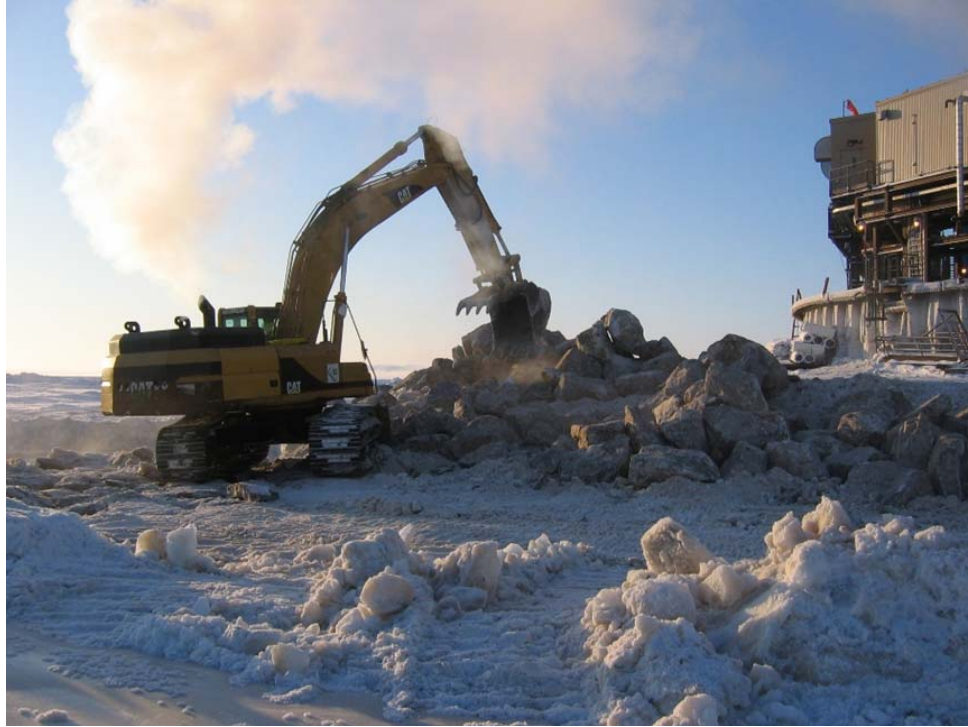
FIGURE A2. A CAT 345B excavator placing boulders at the northeast corner of the Island.
