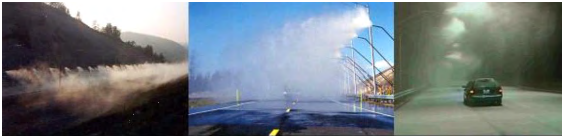
Figure 64. Fog, Rain, and Snow Equipment Installed on the Smart Road
