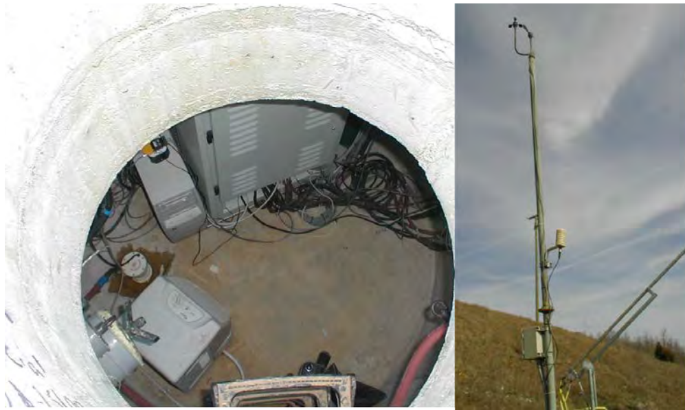
Figure 66. Bunker With DAS and Weather Station Installed on the Smart Road
