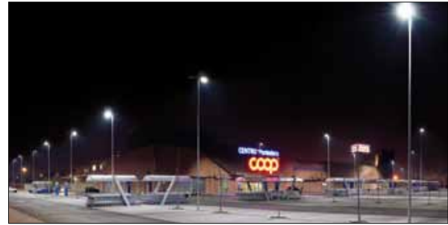
An outdoor lighting installation at Coop Pontedera in Pisa, Italy, showcases Ruud Lighting's BetaLED technology. The company was one of the winners of this year's E Awards. (photo ©2011 Ruud Lighting, Inc. (BetaLED))
